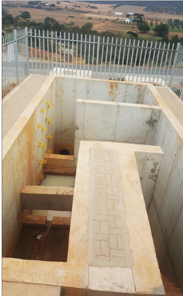
Figure 5: Litter Trap for trash and pollution control
