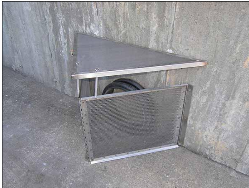
Figure 11: Stormwater Debris Screen device
