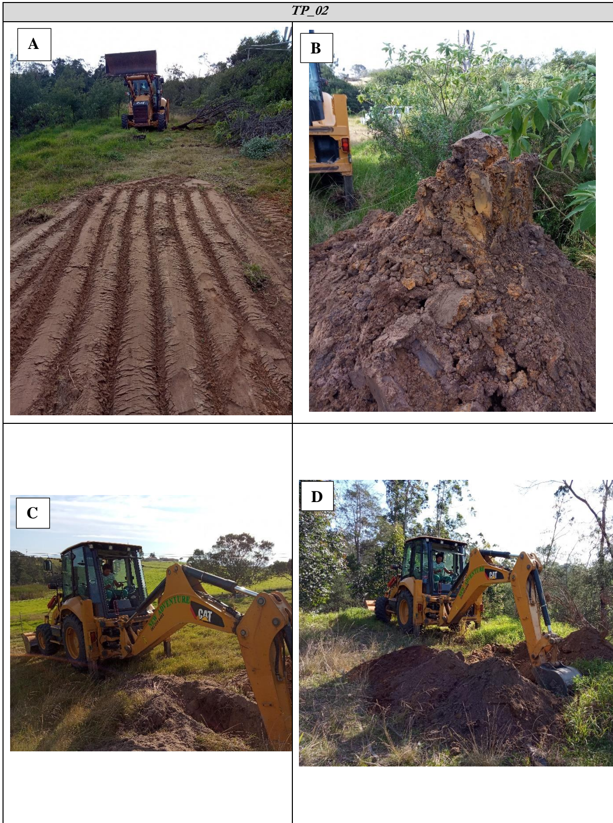
Figure 8: A shows TP3 backfilled and levelled, no sign of collapsing soils, B shows mounding of the stiff clay in TP4, keeping the shape of the TLB bucket, C shows the excavation of TP5 and D shows excavation of TP7 where a package plant is to be constructed.
