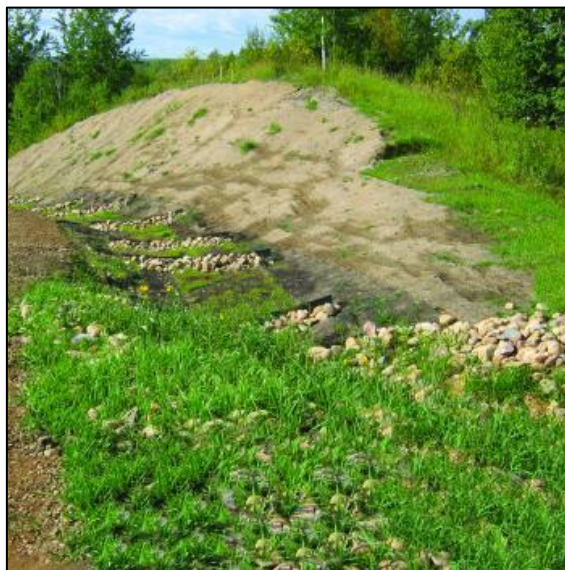
Figure 11: An example of rehabilitation, using various measures to stabilise and recontour a gully, that could be applied to the eroded gully below the dam.
