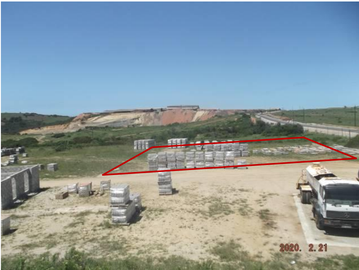
Figure 11: Aerial view of the proposed development site, showing the approximate location of the Depolymerisation Processing Plan in red.
