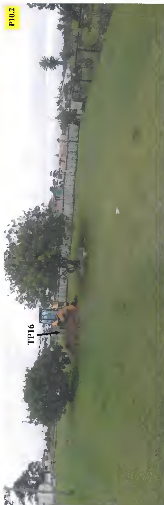
TLB in process of digging TP16 in back garden of House Olivier.
