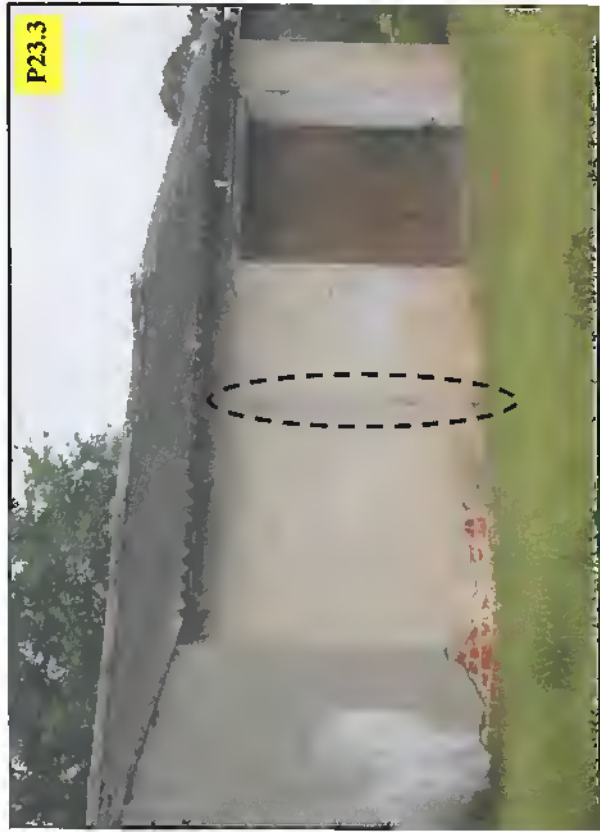
Closer view of vertical crack in north wall of shed shown on P23.2.
