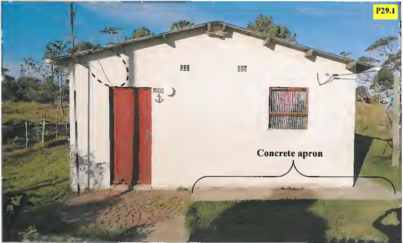
Typical RDP house on the corner of Du Plessis Street and Trekker Road on the north-east corner of the existing housing development. Only southern perimeter of house provided with concrete apron.
