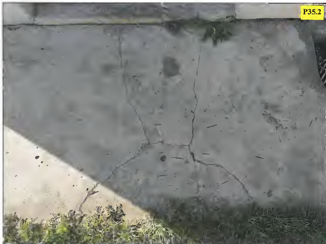
Cracked apron slab at front door.
