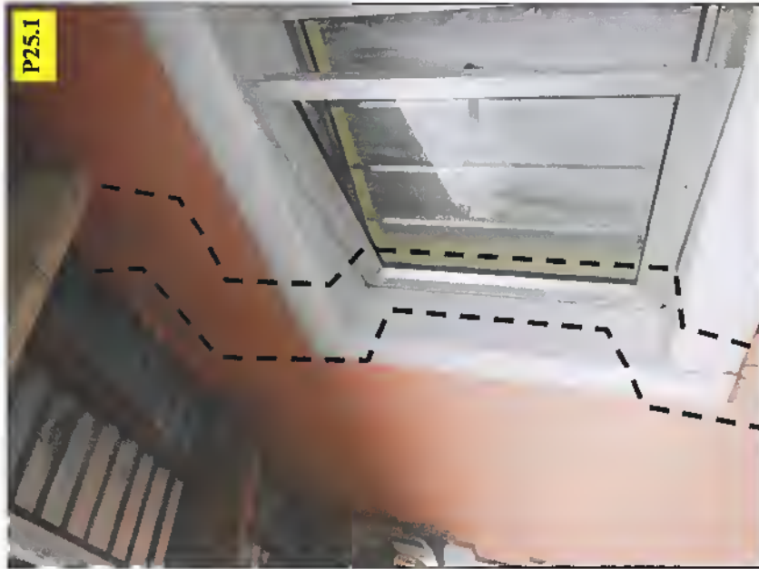
Vertical crack approximately following the movement joint shown on photo, P25.3.
