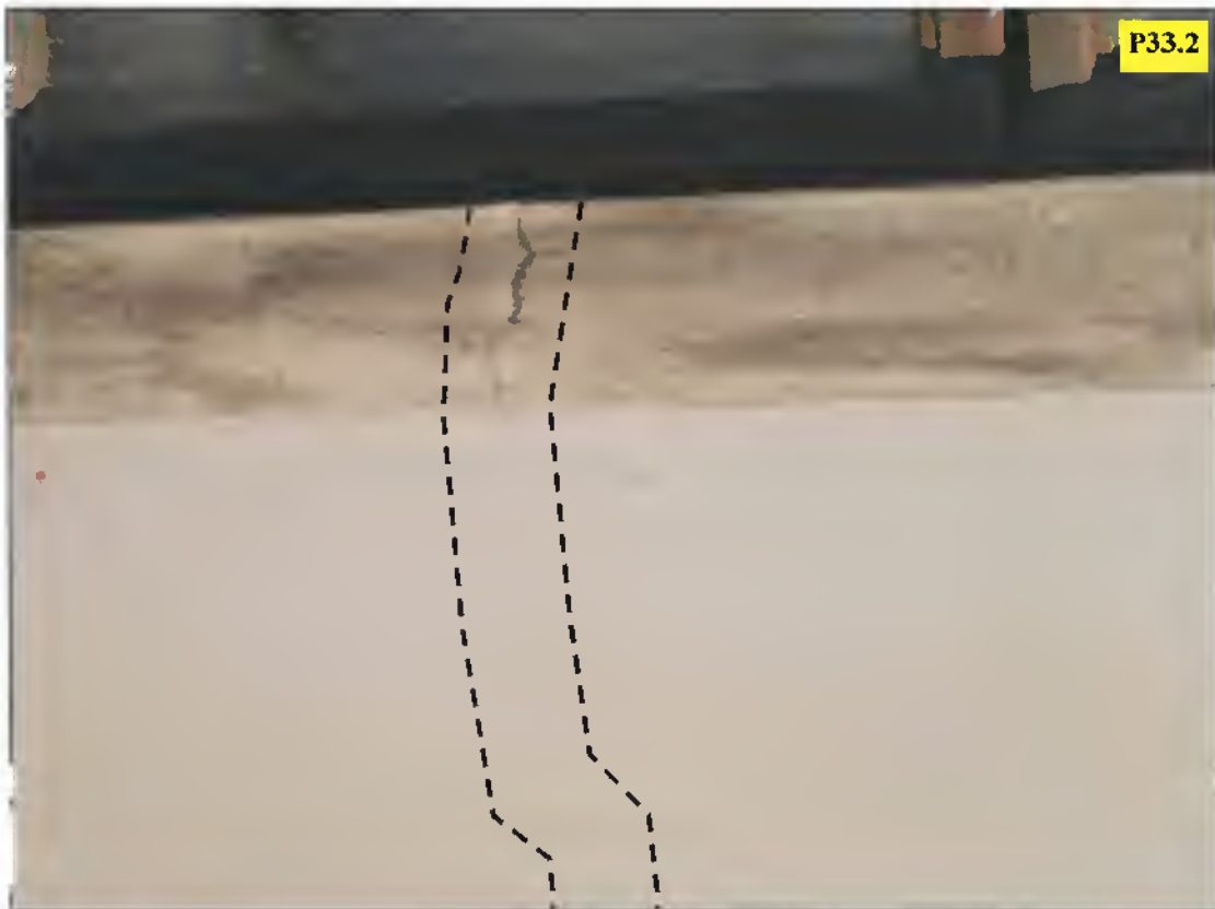
Close-up of above crack extending through window sill.
