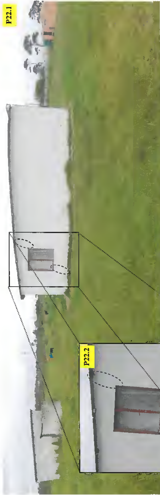
Outbuilding on south-eastern part of Ms Stella Olivier's property. Close-up of outbuilding and crack extending diagonally across side window; note thick kikuyu grass covering surrounding area.
