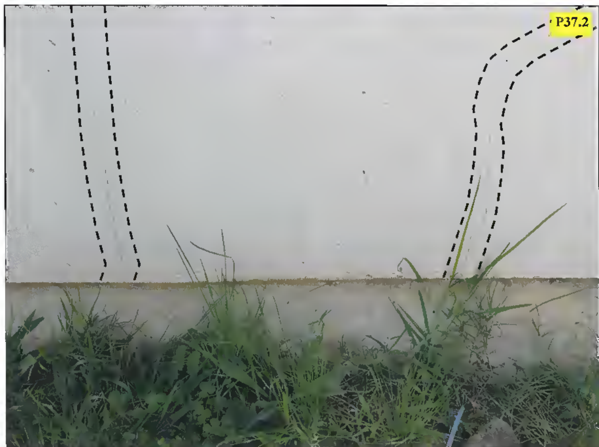
Near vertical cracks and diagonal crack extending from raft foundation to window sill.
