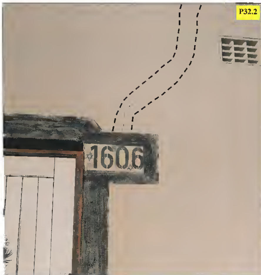
Typical heave-related diagonal crack extending from top corner of front door to the roof.
