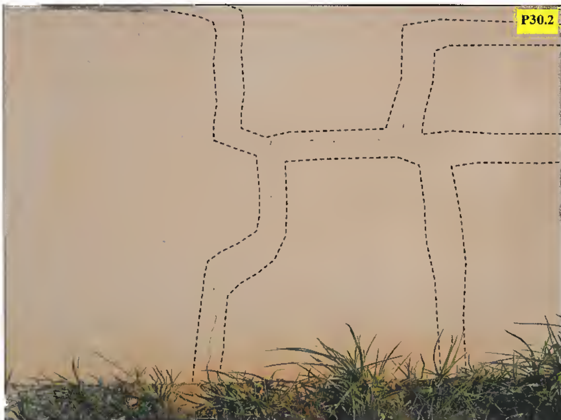
Rectangular cracks, the horizontal portions of which appear to follow mortar joints containing brick-force. The pattern of cracking suggests that the walls have been constructed with of cement blocks.
