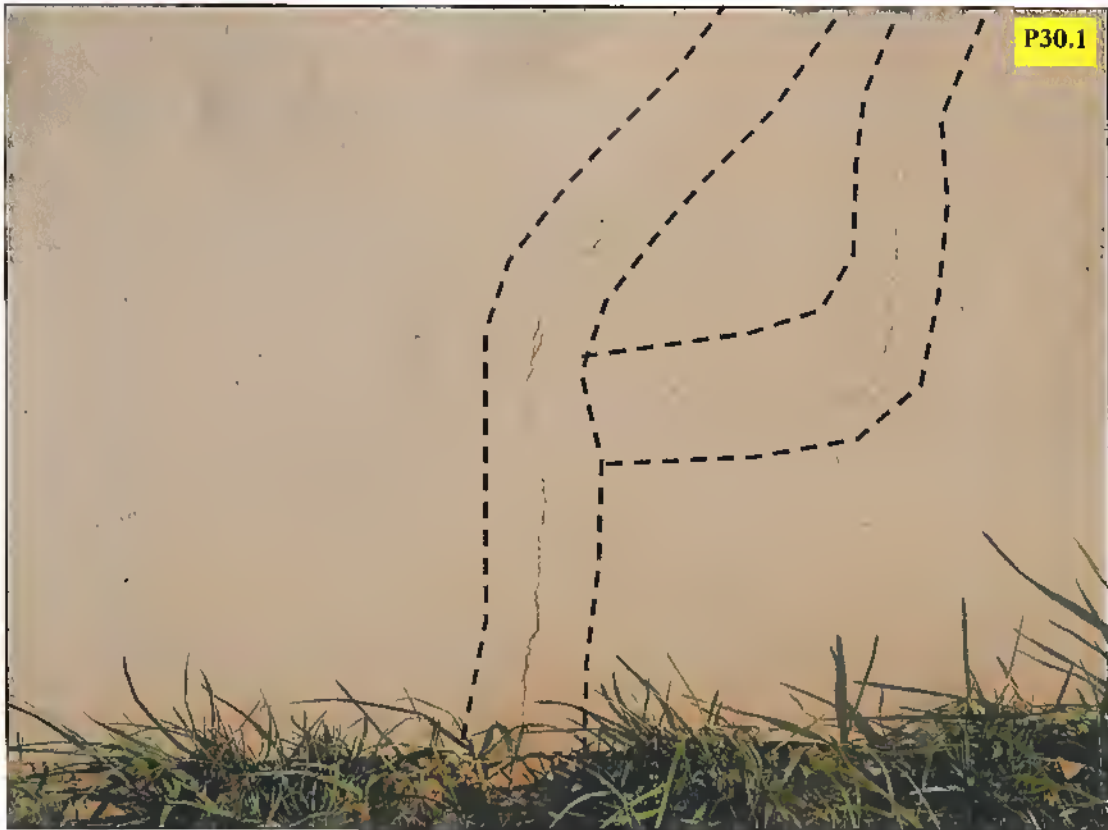
Typical foundation-related cracking occurring mainly in the central parts of the gable ends of the houses.
