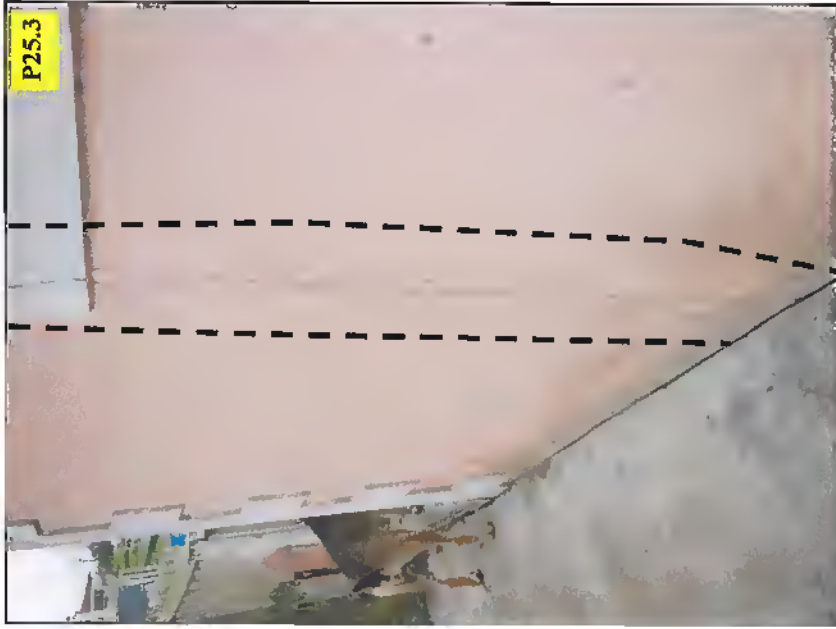
Continuation of crack beneath window shown on photo P25.1.
