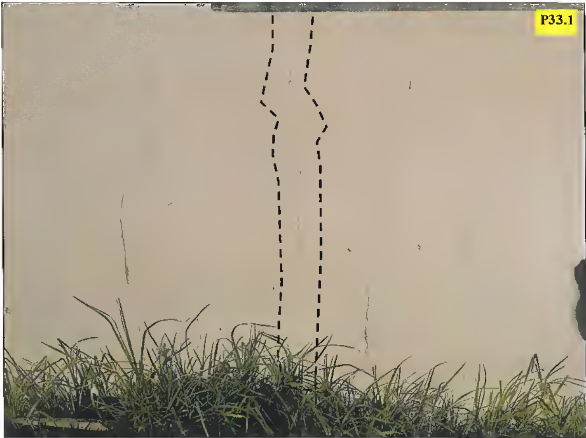
Vertical crack extending from the, apparently raft foundation to the window sill.
