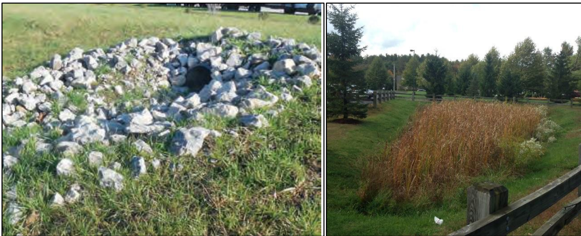
Figure 16: Examples of erosion protection and pollution control measures for consideration in pit water discharge management through the existing stormwater drain towards the wetland.
