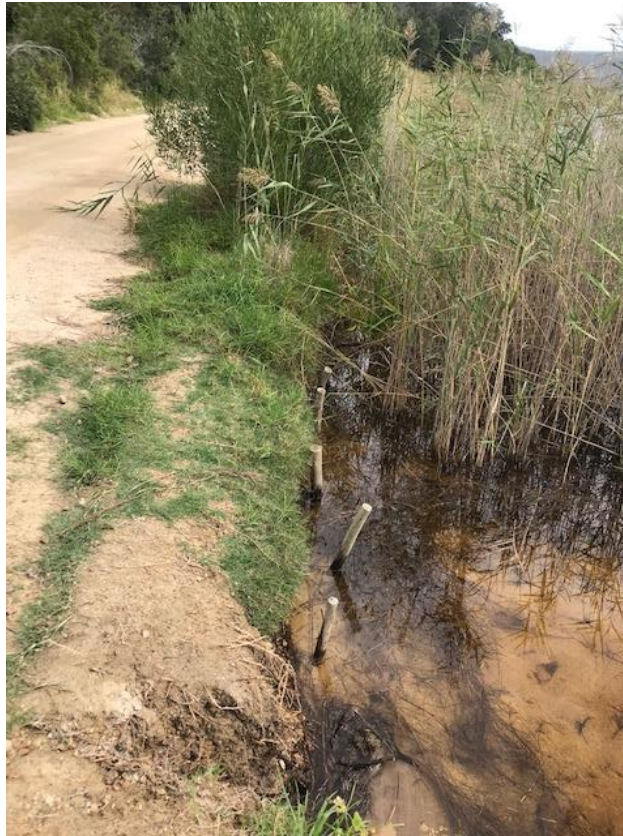
Figure 10. Section of the road where sandbags were historically placed but have now disintegrated allowing erosion to recur.
