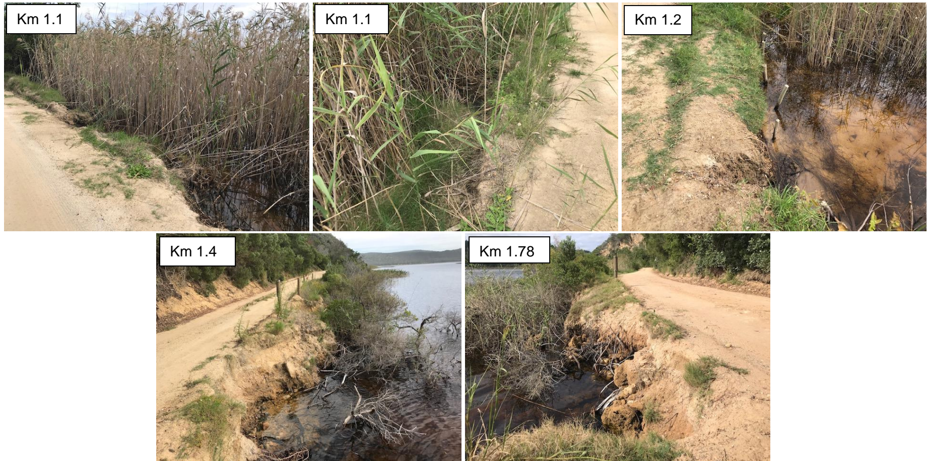
Figure 11. Photos showing various sections of the road OP06914 where erosion is occurring taken 24 March 2021. Kms measured from the N2 highway.
