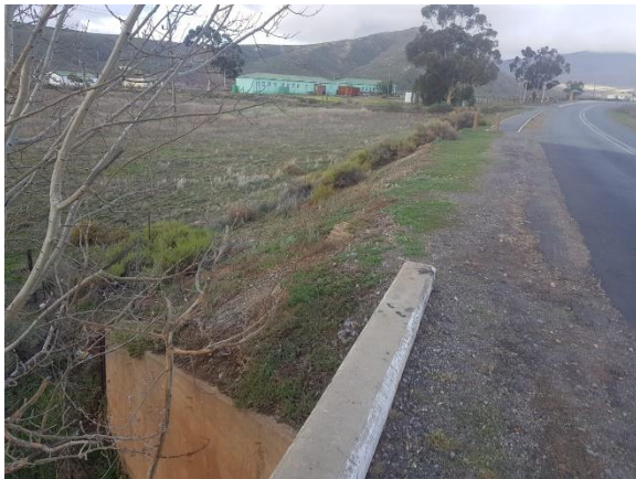
Image 26: Disturbed area adjacent to Major Culvert C10508.
