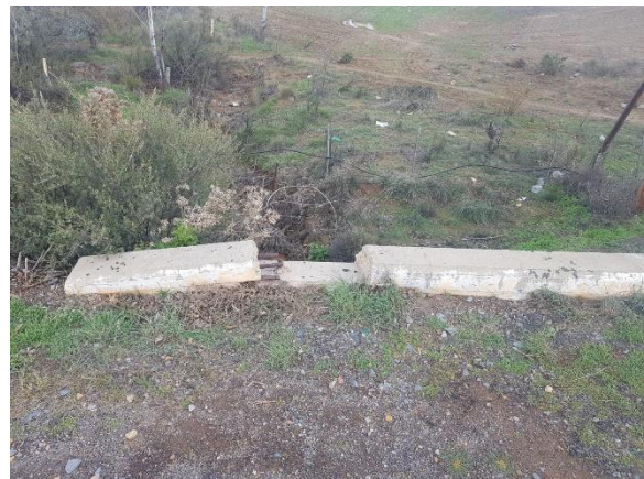
Image 21: Damaged infrastructure on Major Culvert C10508.
