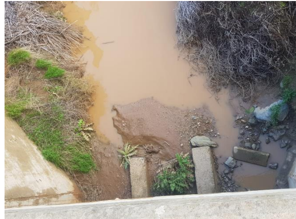
Image 13: Silt within the watercourse.
