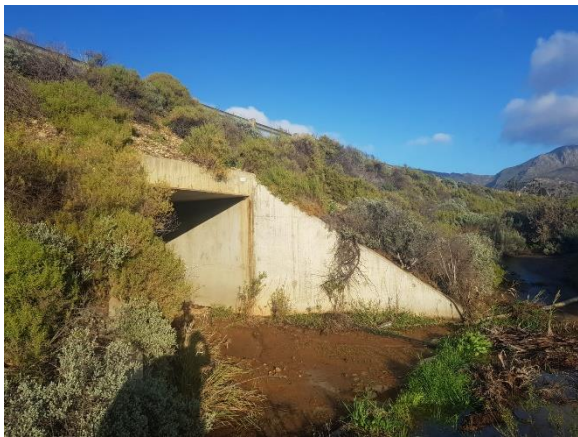
Image 87: Western flow path and steep gradient.
