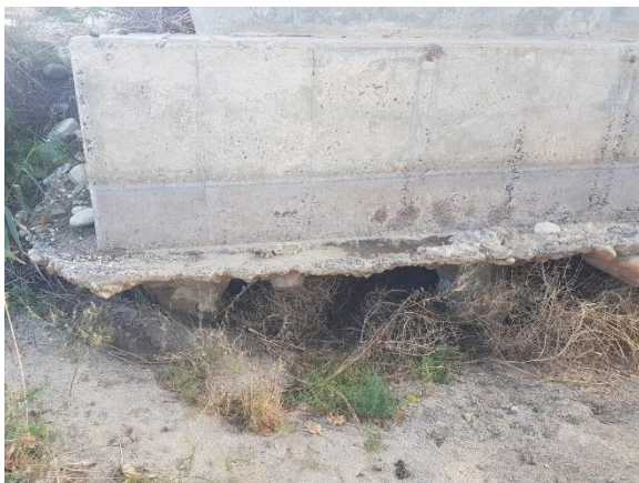
Image 60: Erosion underneath infrastructure.
