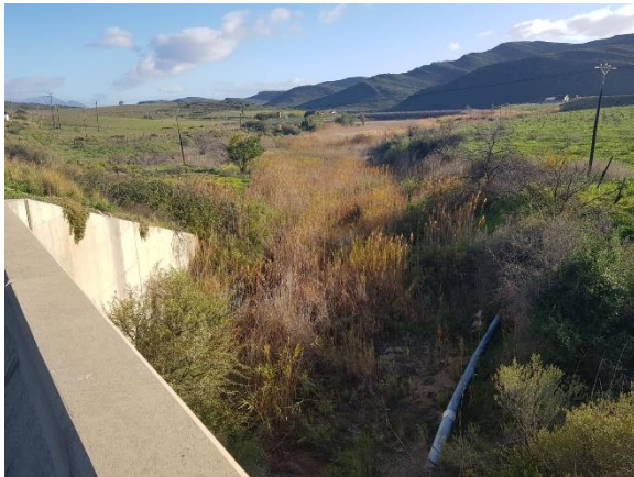
Image 118: Piping infrastructure within flow path.
