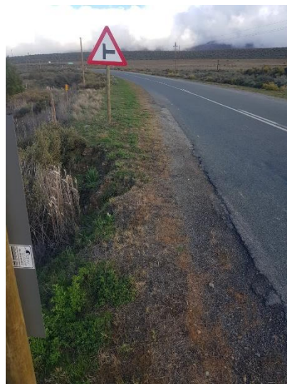
Image 10: Disturbed and erosion area near the Koo River Bridge.
