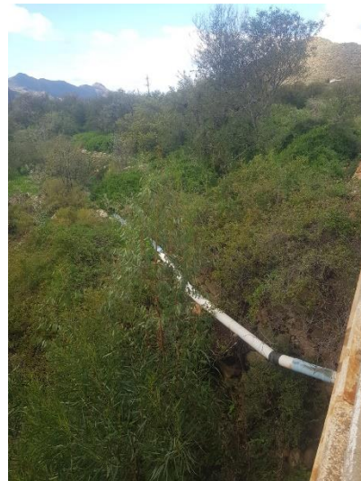
Image 50: Piping infrastructure on the Keisie River Bridge.
