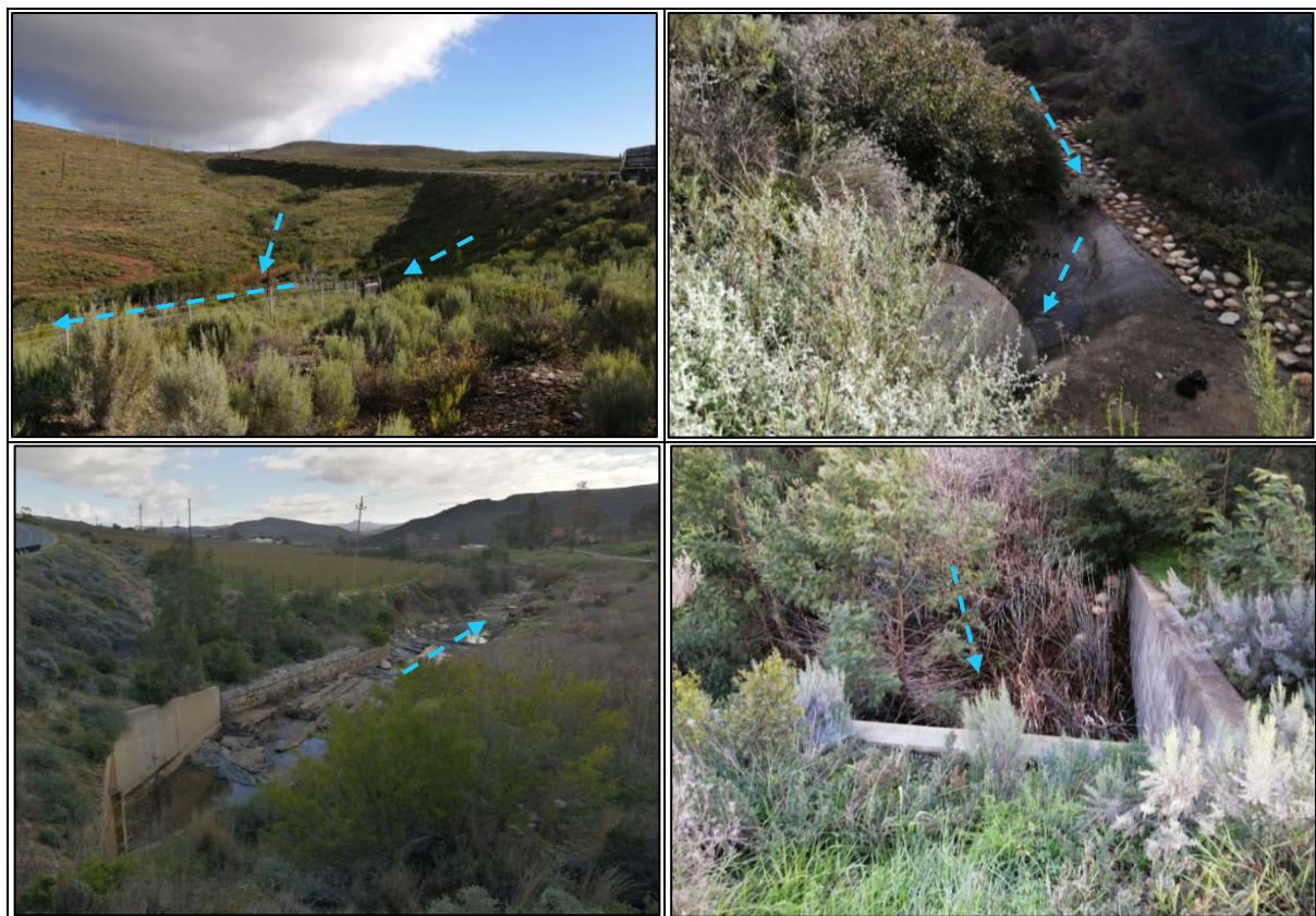
Figure 49: Photographs of culvert structures along the road which require normal maintenance work, such as clearing the flow paths
