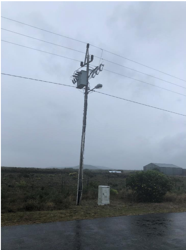
Figure 2: Existing 50kVA Pole-mounted transformer & kiosk
