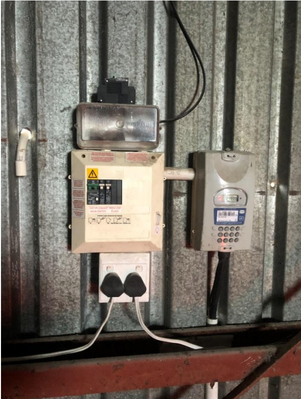
Figure 3: Existing Electrical DB and Pre-paid Meter
