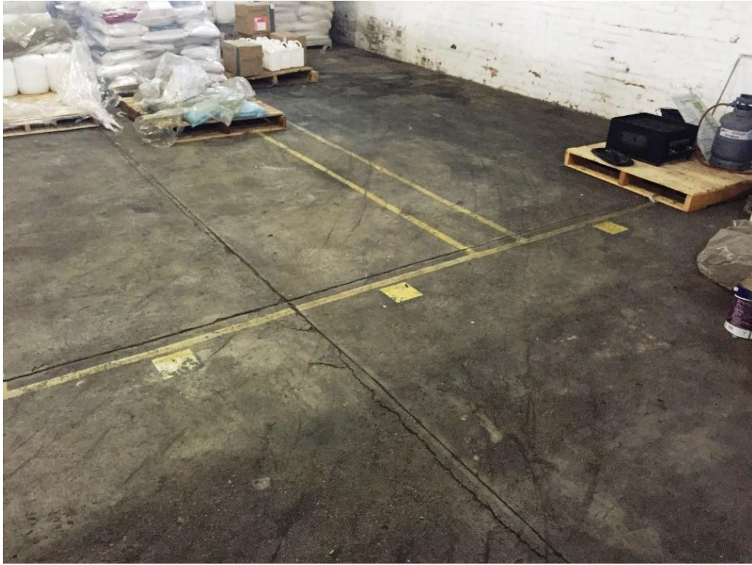
Photo 5: Warehouse Floor B - notice edge breaks
