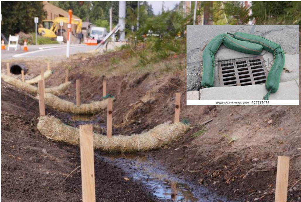
Figure 19: Examples of silt socks placed perpendicular to the flow of water. These reduce the force of water flow, erosion, and can prevent unwanted sedimentation on the site.
