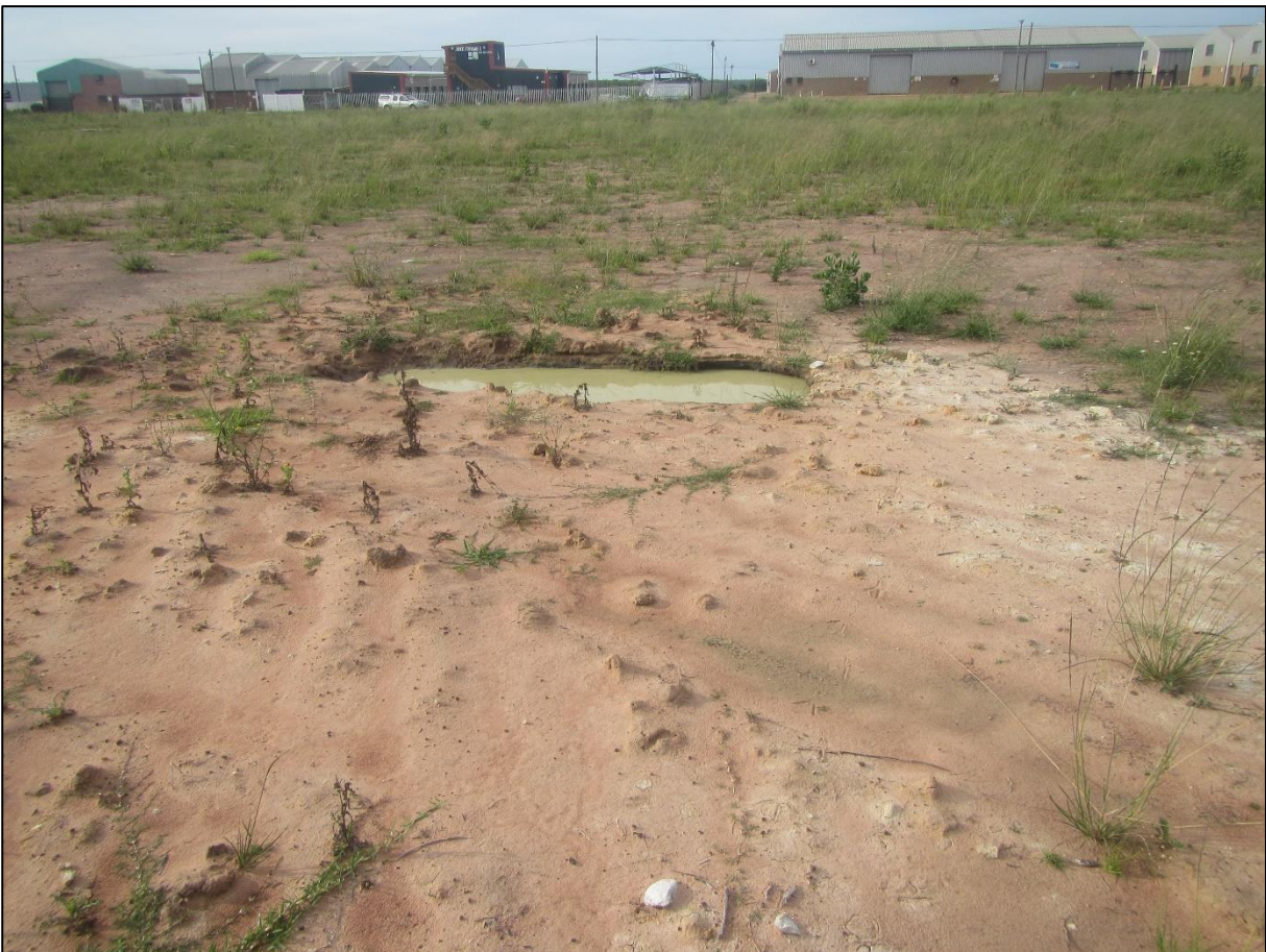
Geotechnical excavation in the centre of the site revealing a clay substrate.
