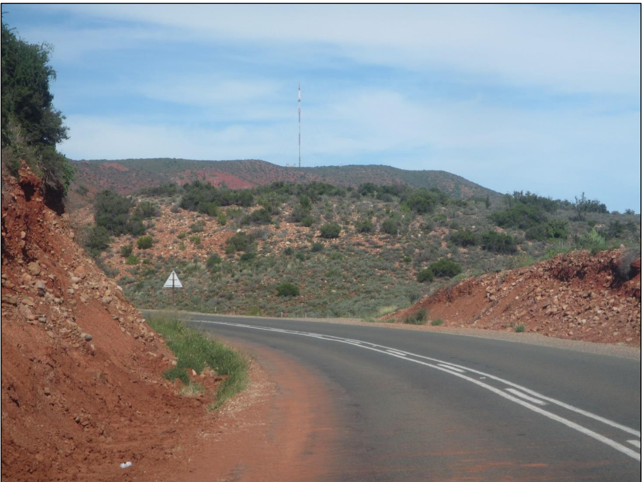
Figure 13: View looking southbound showing a slightly unstable road cutting.
