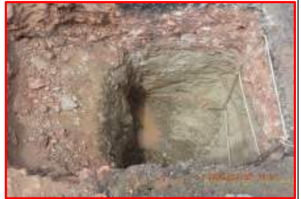
Water infiltration @ 0,7m (next to V-Drain)
