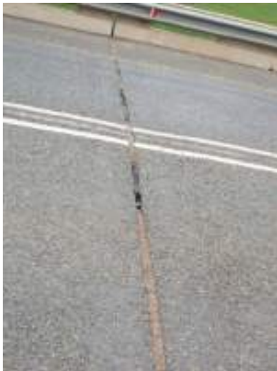
Joint condition prior to 2008 seal installation.
