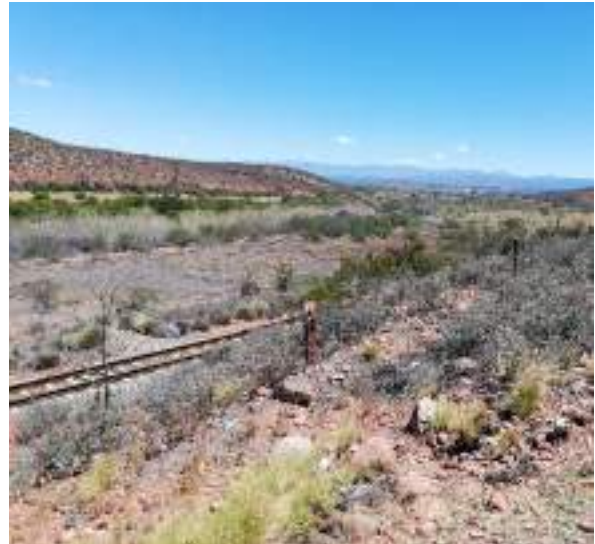
Photo 13.2 MISSING FENCE BETWEEN KM 28 AND KM 29 ON LHS OF THE ROAD
