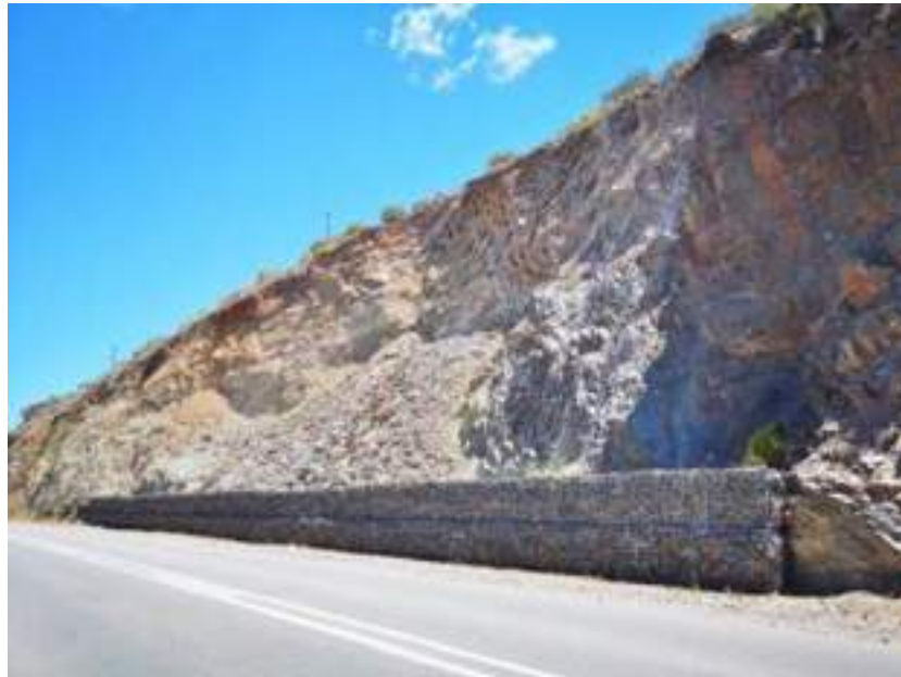
Photo 4.2 MESH DRAPERY SYSTEM AND GABION WALL AT KM 23.0
