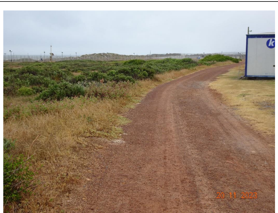
Figure 2 – Condition of Northern access road.
