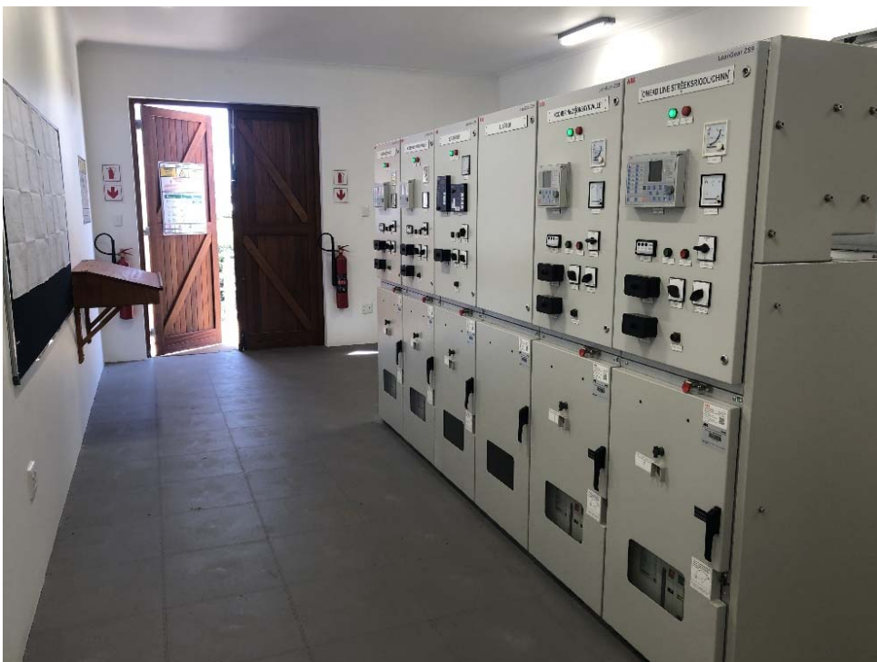
Figure 4-19: Typical MV Substation Building (Internal)
