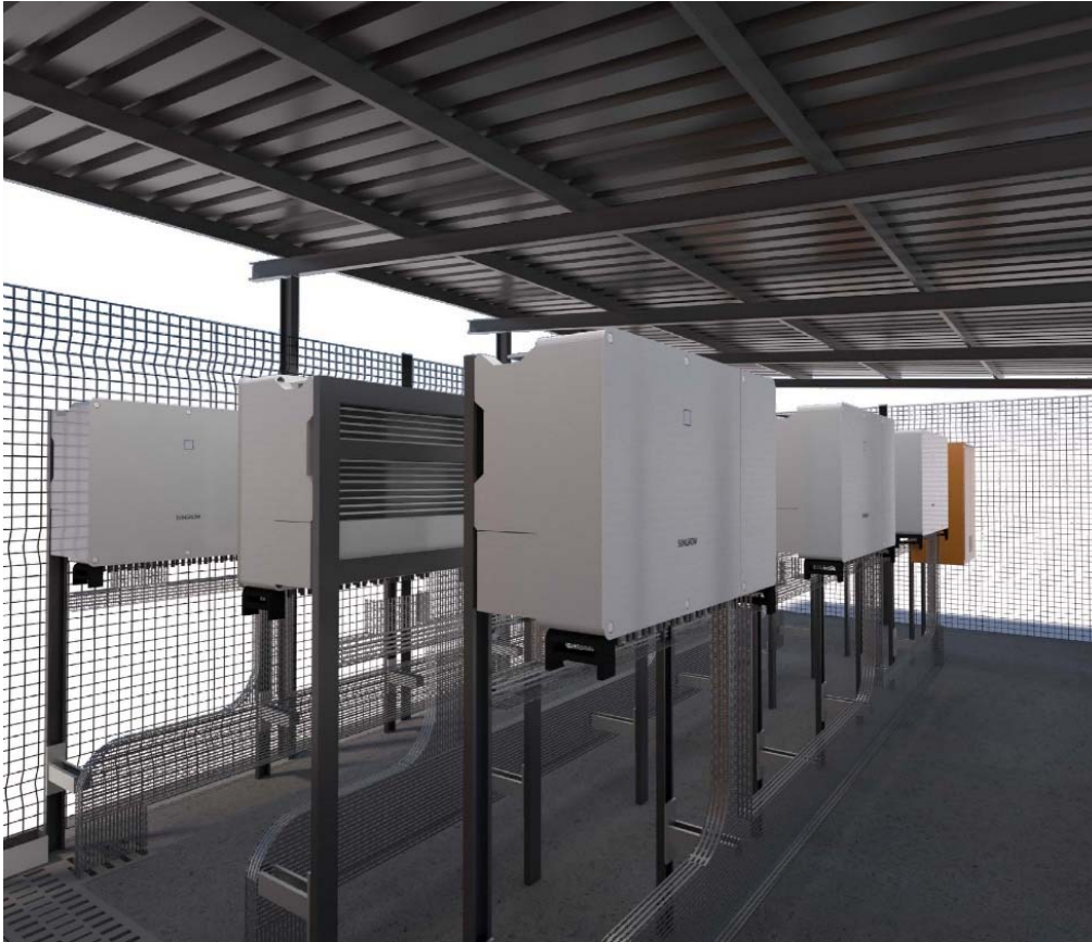
Figure 4-14: Inside of String Inverter Canopy (Credit: Eversolar)
