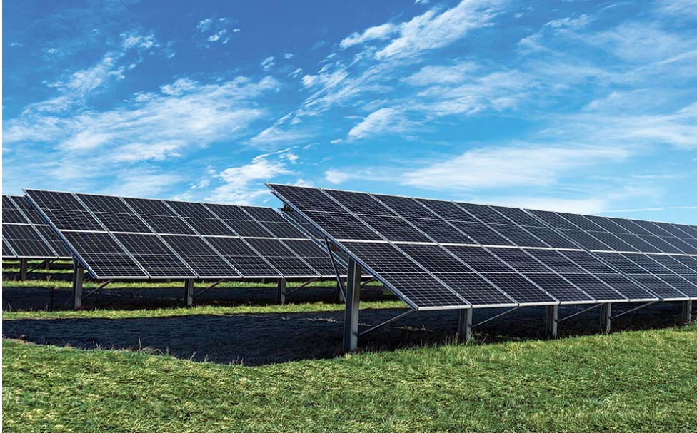
Figure 4-11: Typical Fixed-tilt Ground-mount System (2V Arrangement)
