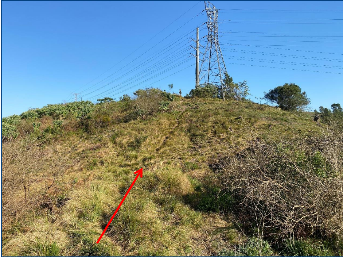
Figure 5-5: Close-up view of the middle section of pipeline route, populated by grasses and bugweed.
