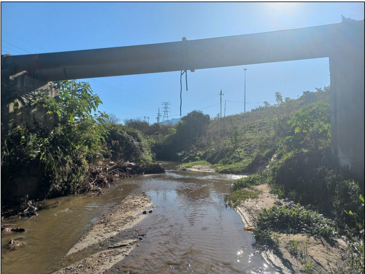
Plate 4: Photograph showing the degraded state of the river system, with erosion and deposition clearly evident, alien invasive plants, and indicating the pipeline crossing and stormwater outlet
