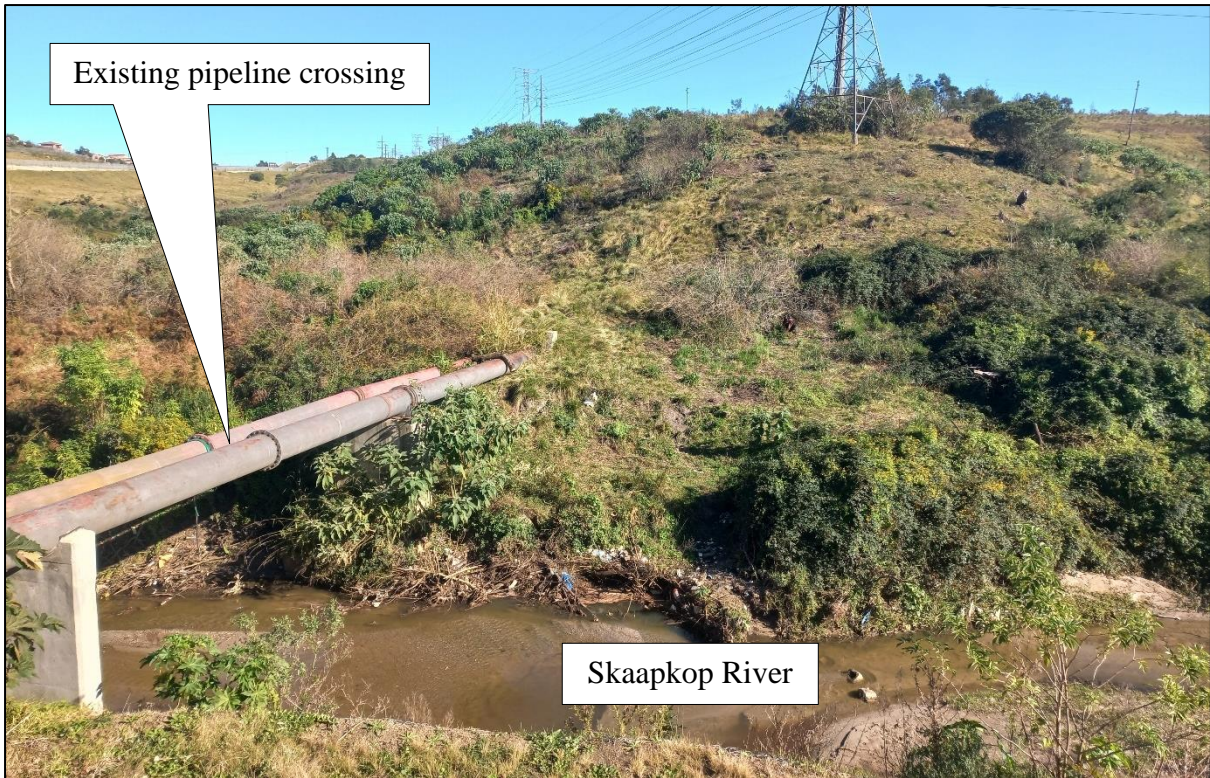
Plate 1: Photograph of the existing sewer pipeline crossing, from the pump station across the Skaapkop River, which requires upgrading.
