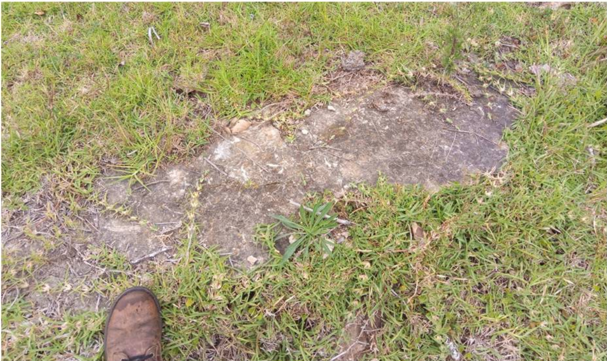
Figure 30. Example of stone wall footing in quartzitic sandstone (top) and cement/concrete slab / floor (bottom). Hand and boot for rough scale.
