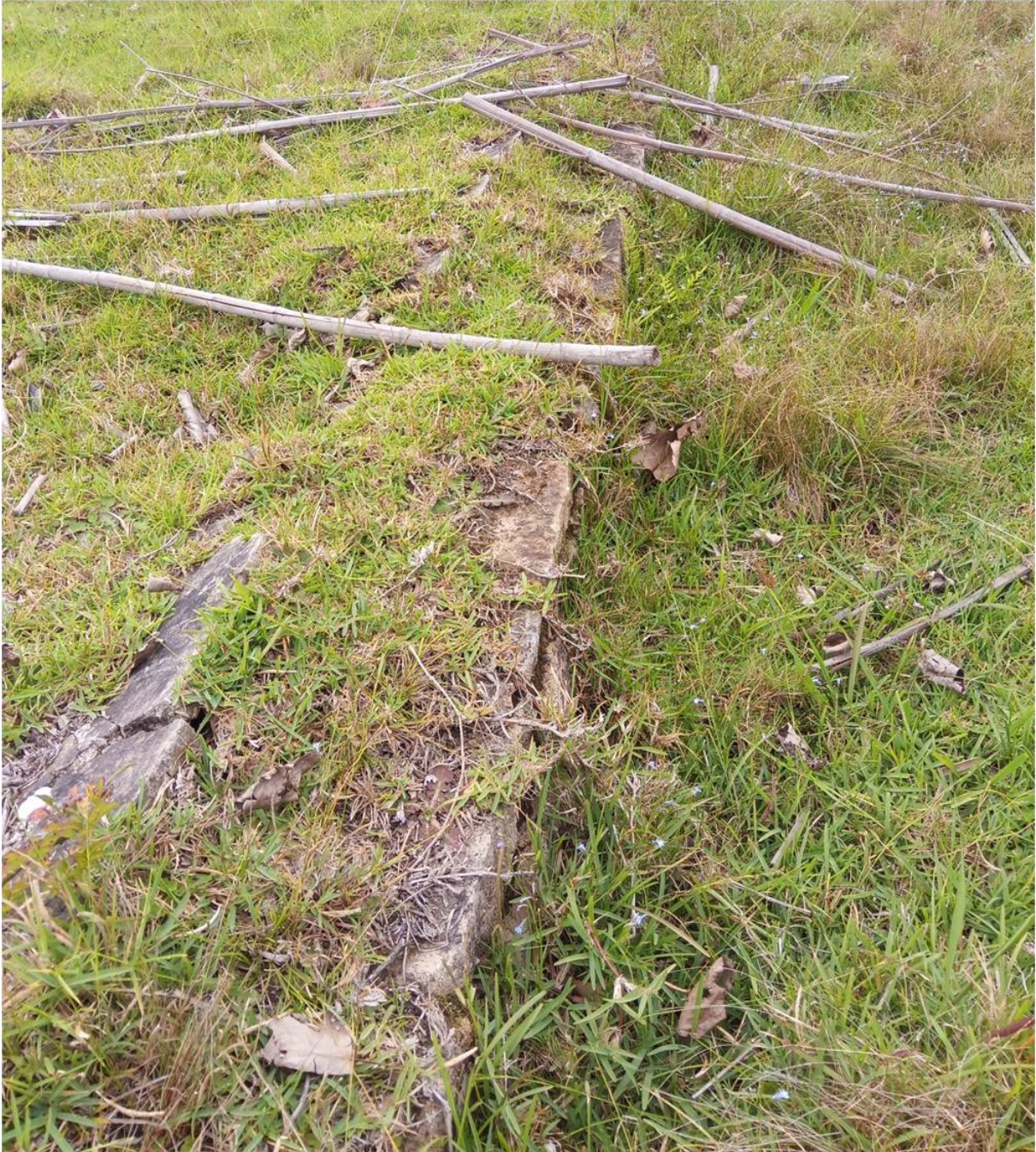
Figure 29. Example of stone wall footing and collapsing cement/concrete slab (left of stone wall footing).
