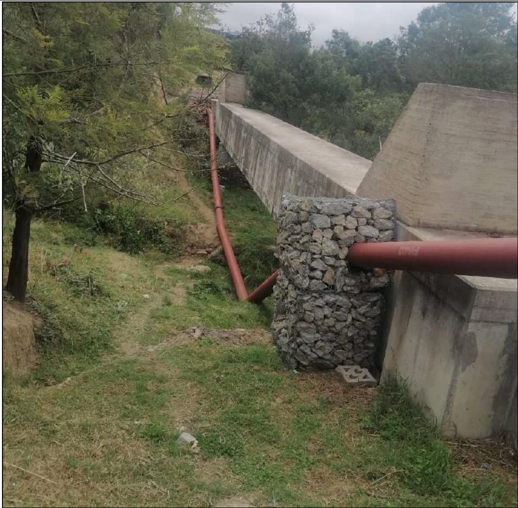
Figure 22: Alternative A, Preferred Alternative (example of a typical u channel concrete pipe bridge)
