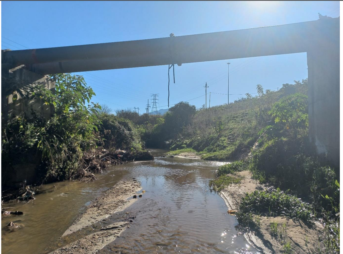
Figure 17: Photograph showing the degraded state of the river system, with erosion and deposition clearly evident, alien invasive plants, and indicating the pipeline crossing and stormwater outlet.
