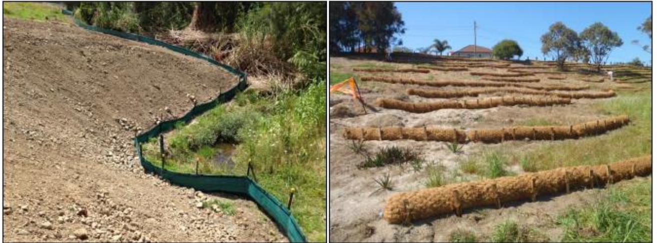
Figure 22: Examples of silt fences (left) and coir logs (right) used to trap sediment mobilised from steep slopes.
