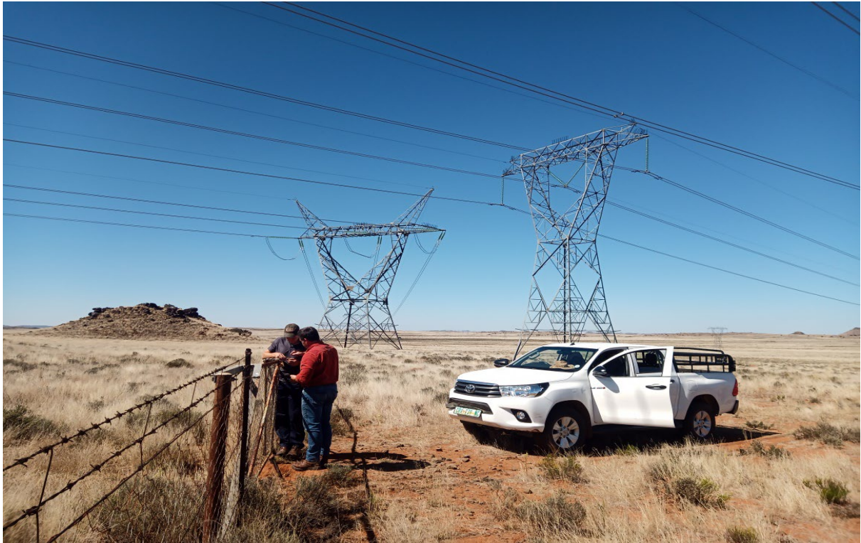
Figure 57: typical farm fence with existing pylons
