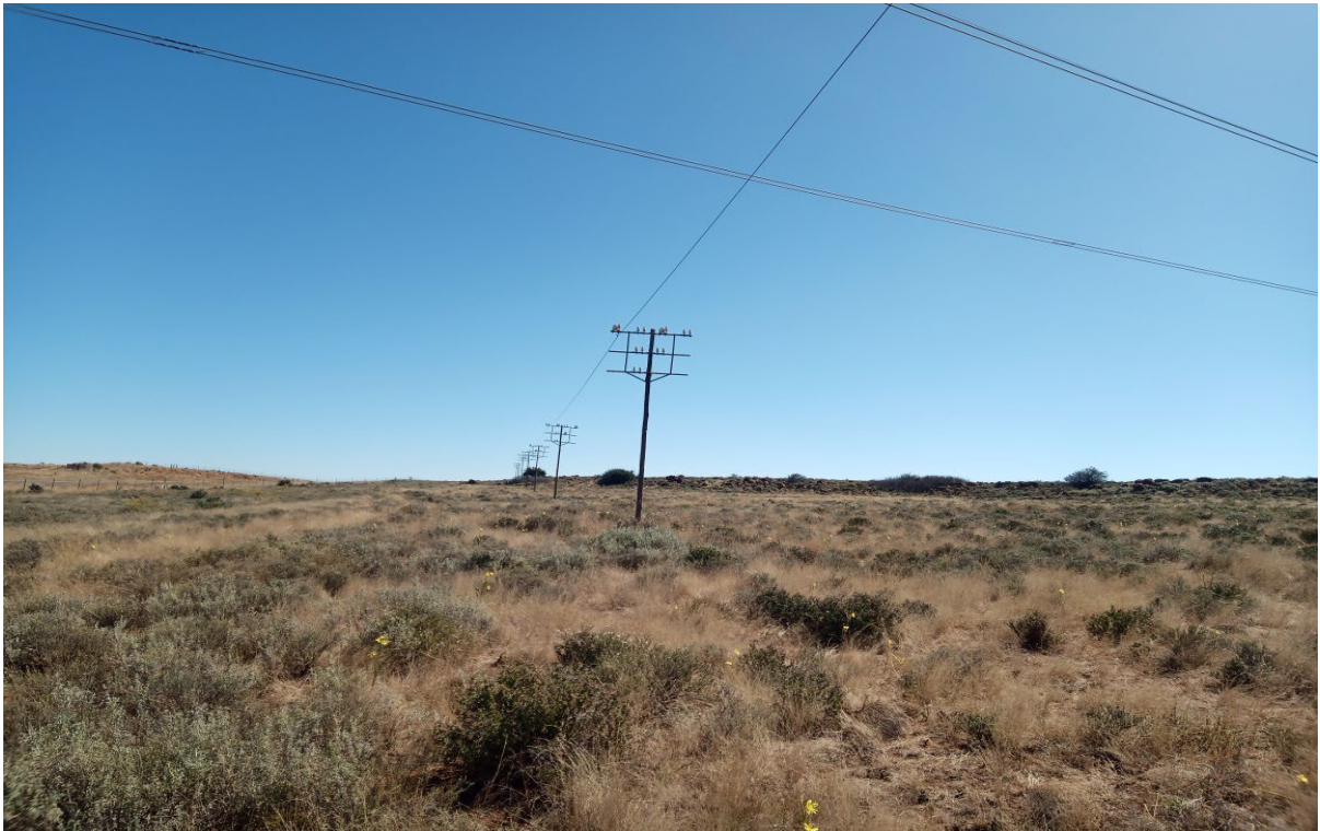
Figure 47: remnant telephone infrastructure
