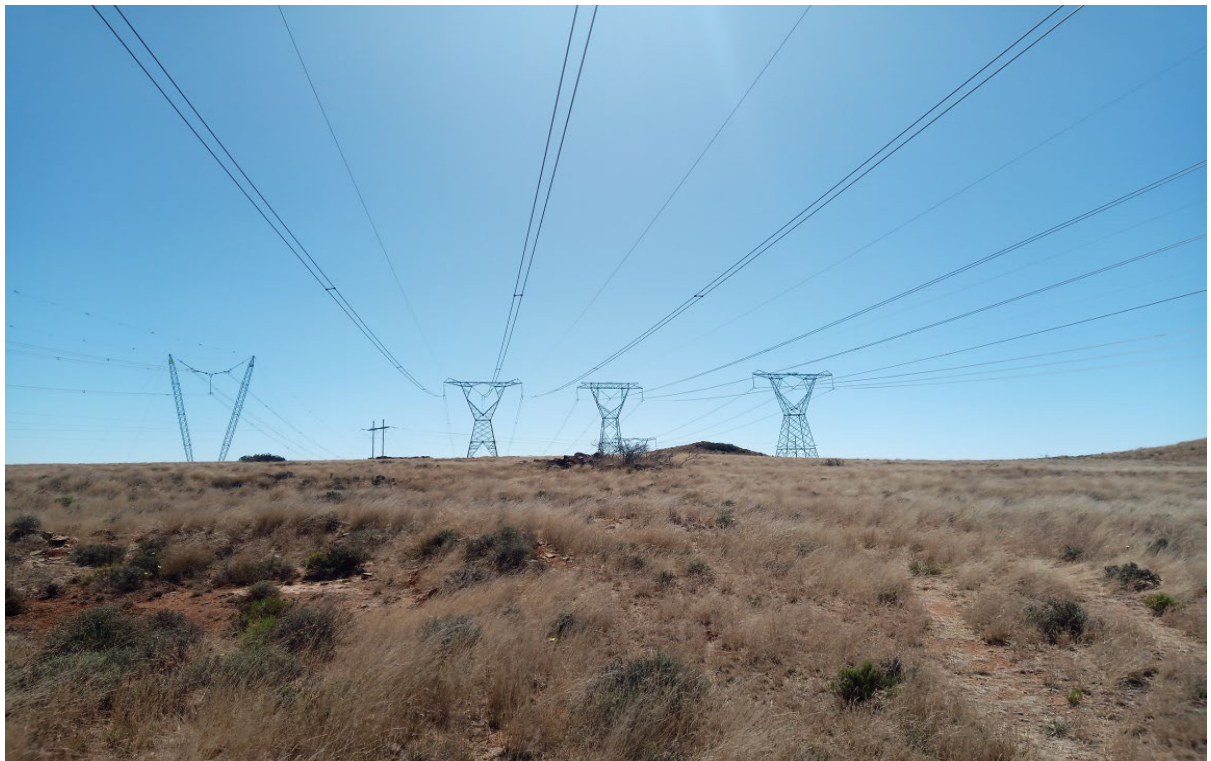
Figure 58: extent of existing powerlines on site
