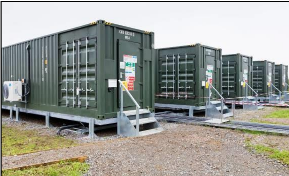
Photograph 1.2: Example of BESS located in storage containers
