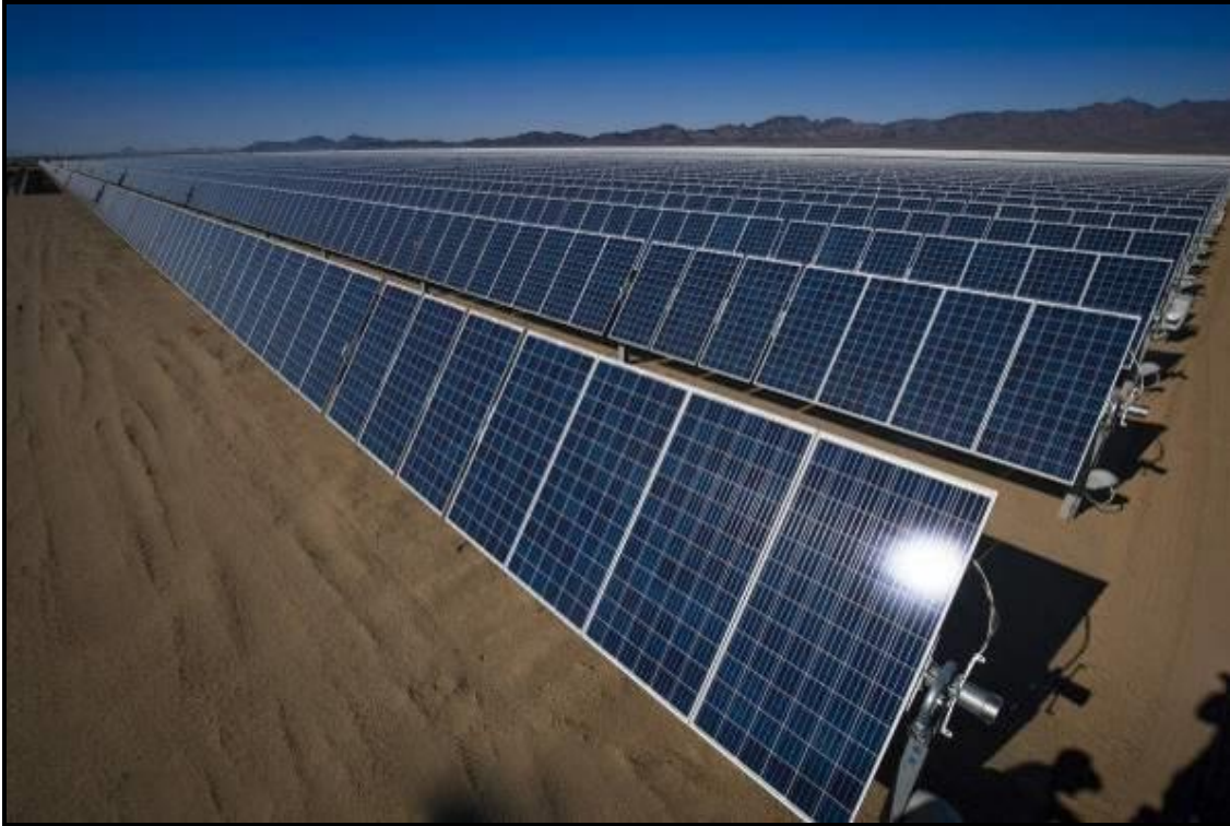
Photograph 1.1: Typical PV SEF facility
