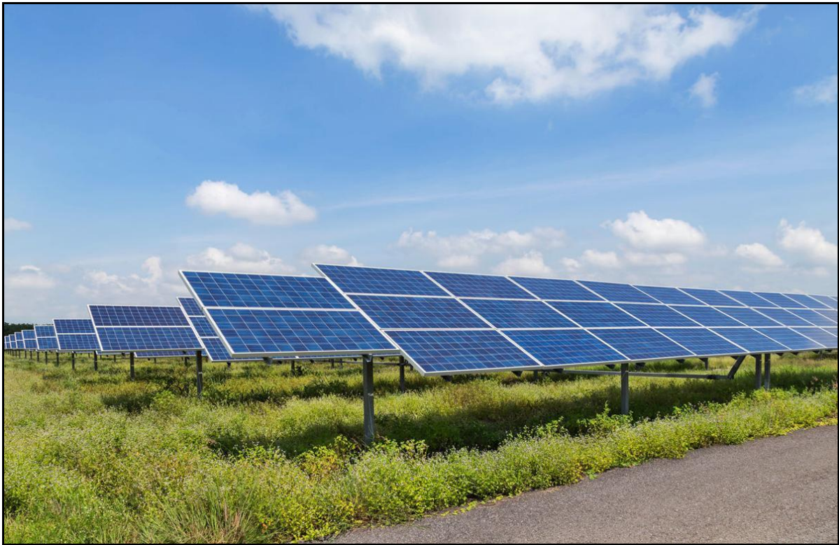
Photograph 1.1: Typical PV SEF facility
