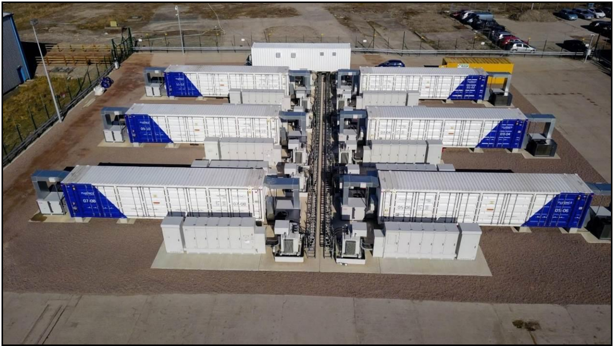
Photograph 1.2: Example of BESS located in storage containers
