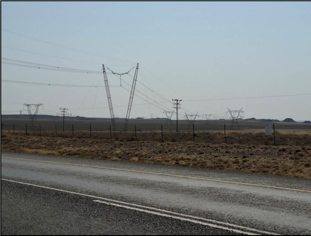
Photograph 3.4: Transmission lines associated with Hydra substation
