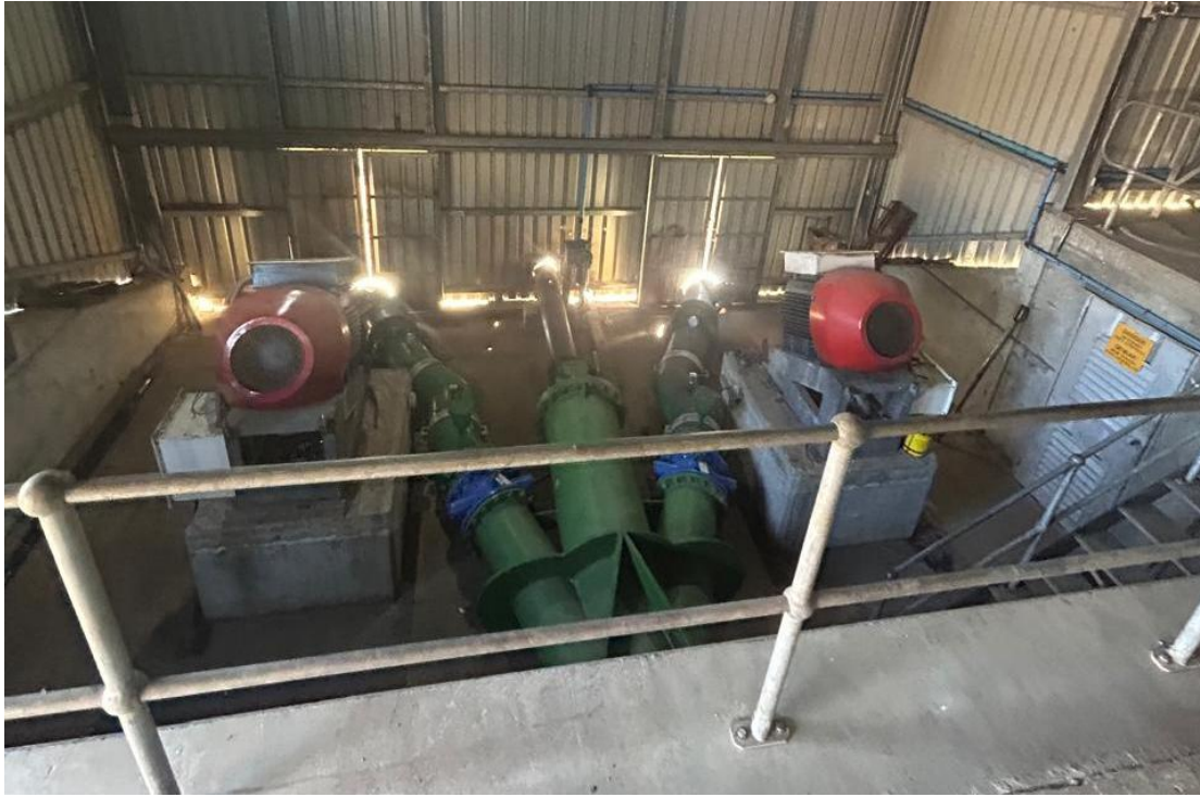
Figure 1-2: Axial flow pump motors
