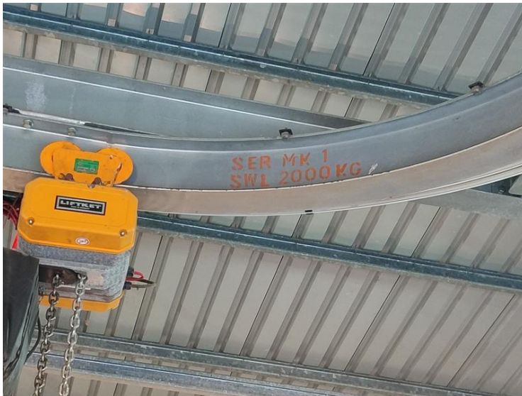
Figure 5-5: Existing pump station hoist
