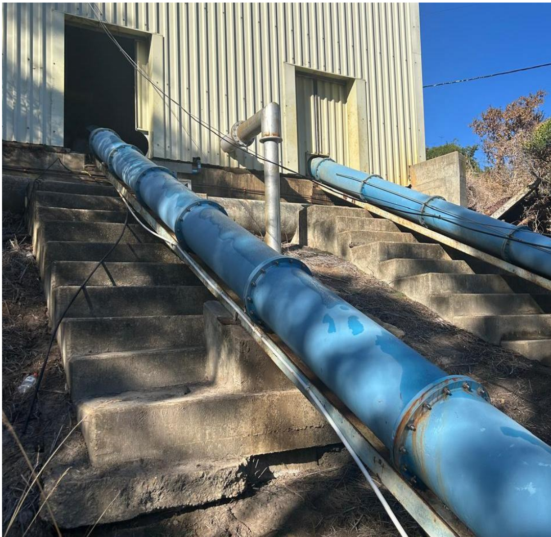
Figure 1-3: Axial flow pump riser pipes/columns
