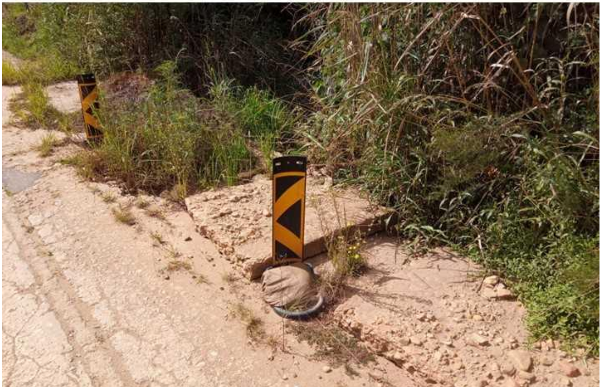
Figure 5. Site 5 showing damage to causeway.
