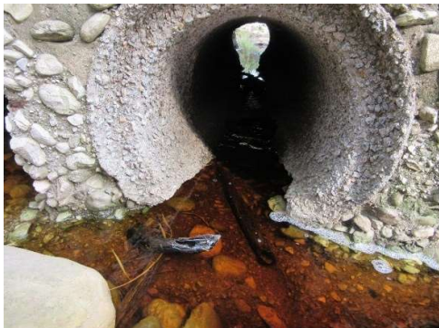
Severe corrosion to invert of pipe culvert
