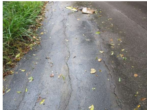
Close-up view of road slip
