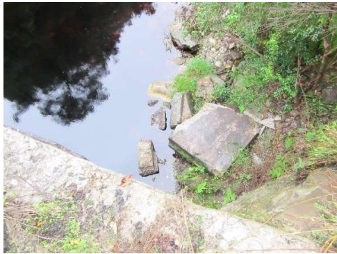
Remains of the damaged end-block and balustrade
