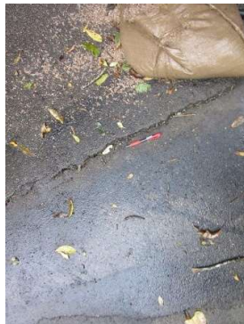
Close-up view of road slip
