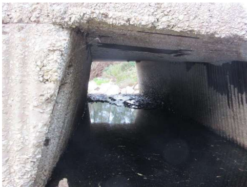
Corrosion visible to inside of causeway structure
