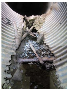
Severe corrosion to invert of Armco culvert
