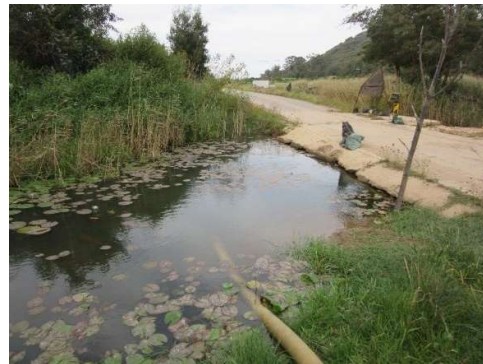
Water ponding downstream of drift
