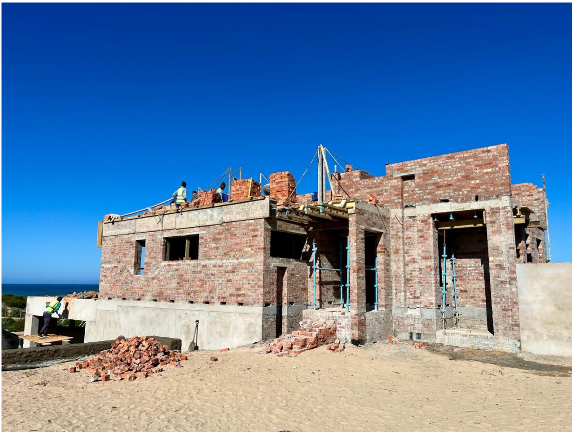
Photo 4: Builder's rubble is to be placed in a skip or stored in a non-sensitive area. This rubble should not be stored on the upper platform but rather on the lower ground level.
