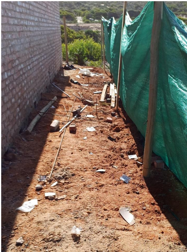
Photo 4: Paper/cardboard tags from the reinforcing steel bars must be picked up and placed in the skip to prevent being blown around the site and onto neighbouring erven.
