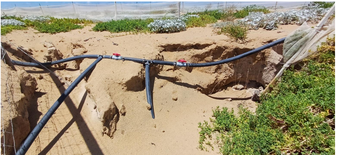
Photo 5: The irrigation pipe pulled out of a fitting and caused some erosion of the rehabilitated dune.
