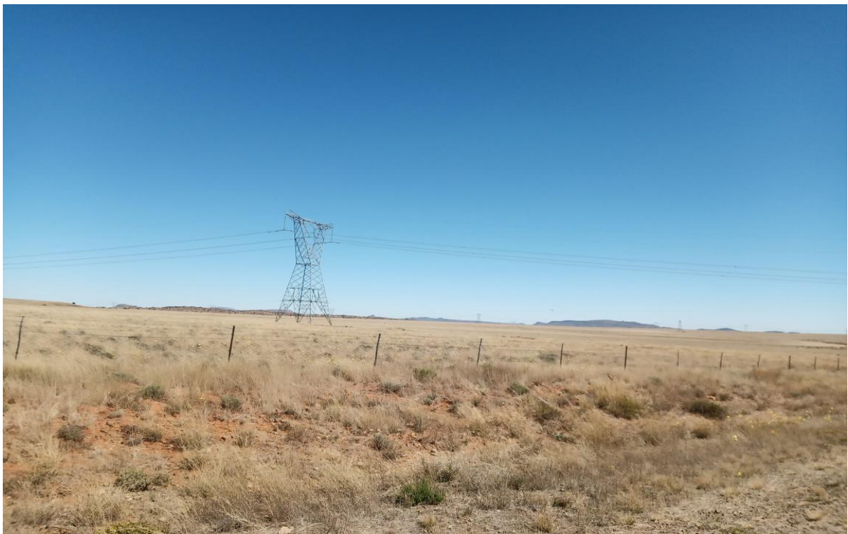
Figure 47: electricity pylons on site
