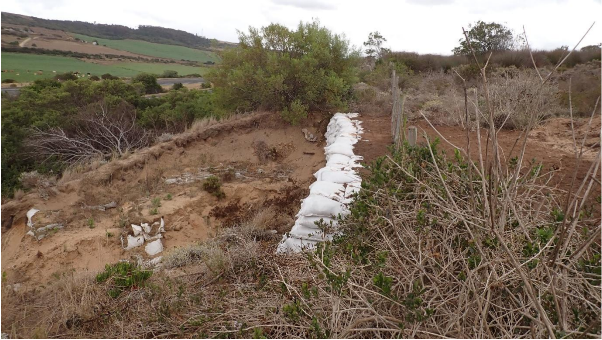
Figure 12: Stormwater management structures across the central area of the property
