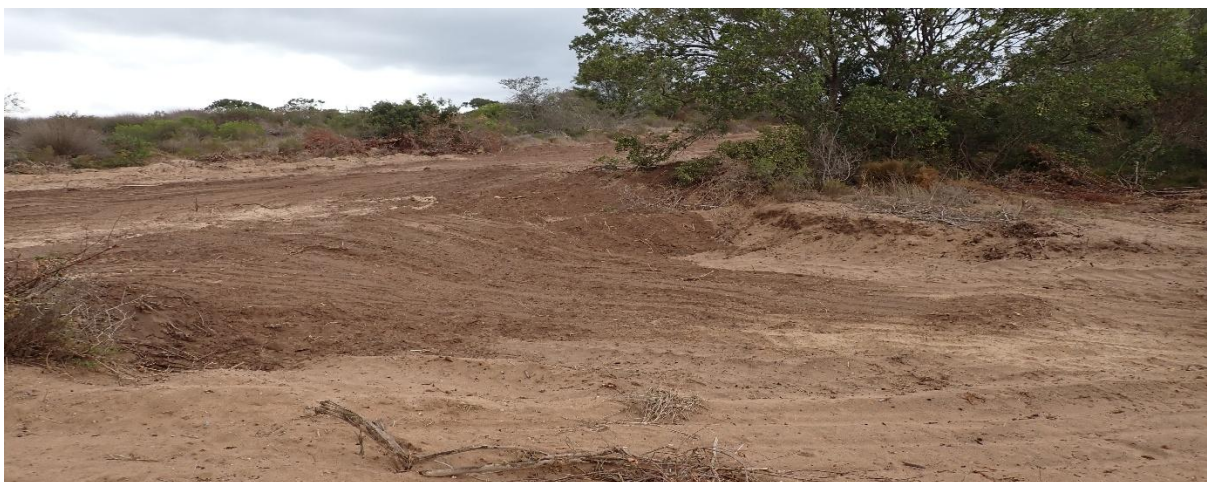
Figure: 12A: Flood damage repairs
