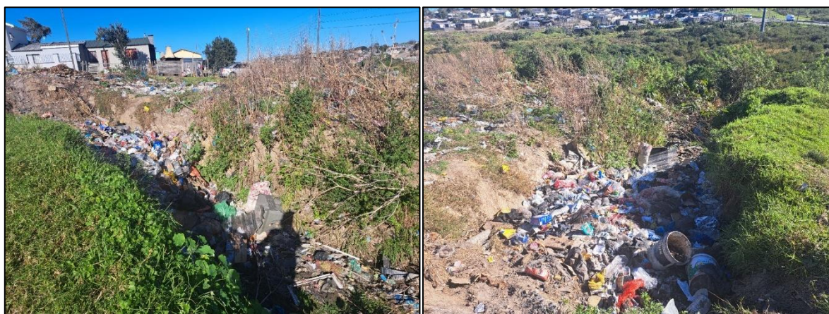
Figure 12: Example of an erosion gully at a stormwater outlet that has become an informal dumping site.
