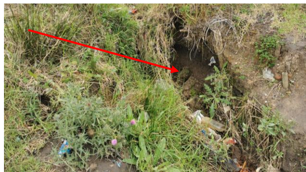
Figure 42: Eroded and polluted watercourse.
