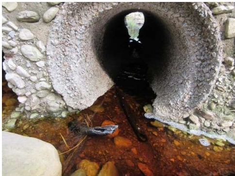
Severe corrosion to invert of pipe culvert
