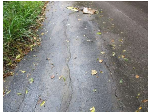
Close-up view of road slip
