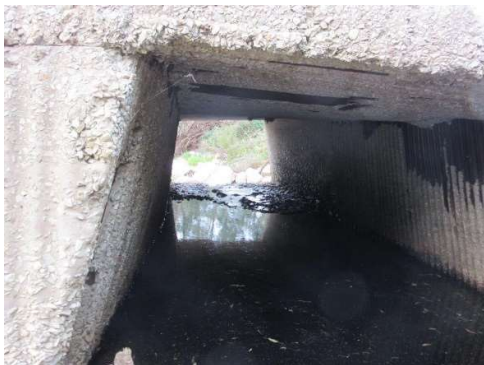
Corrosion visible to inside of causeway structure
