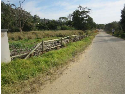
Road DR1791 at km 1.59; upstream on LHS. Debris from previous flood trapped against fence.
