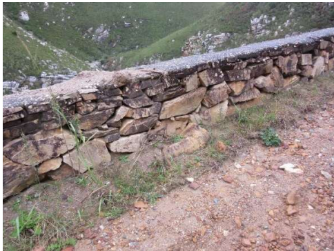
Image of existing dry-stack balustrade wall in Montagu Pass on road DR1640
