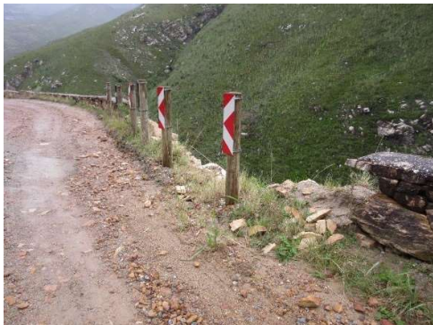
Damage to dry-stack balustrade wall on DR1640 at km 7.63
