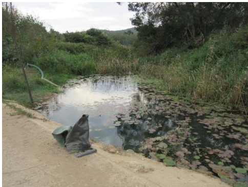
Water ponding downstream of drift
