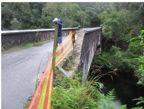
One of the end-blocks and part of the balustrade to the Salt River bridge on road MR00355 at km 8.67 was knocked down by vehicle impact. This is on the RHS when approaching the bridge from Saasveld side.
