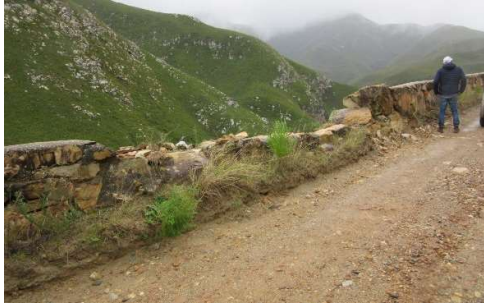
Damage to dry-stack balustrade wall on DR1640 at km 7.87
