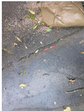
Close-up view of road slip
