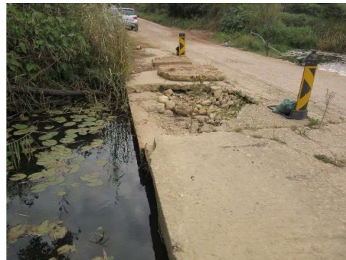
Water ponding upstream of drift. Damage to deck caused during previous flood.
