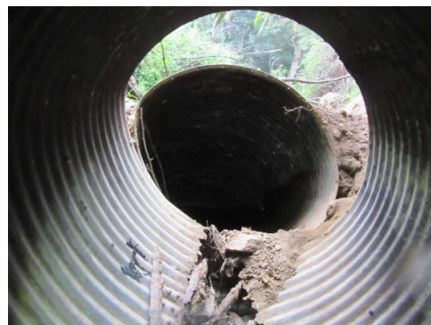
Downstream section of the Armco culvert washed away and collapsed due to erosion
