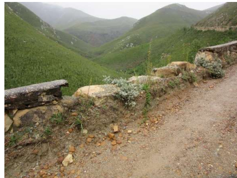
Damage to dry-stack balustrade wall on DR1640 at km 7.87
