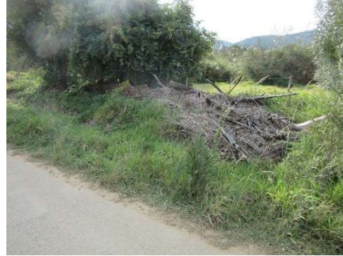
Debris from previous flood trapped against fence on downstream side of road.
