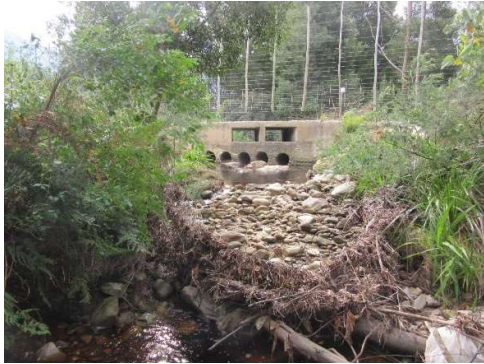
Downstream – looking towards culvert. Flood fence missing.
