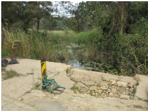
Water ponding upstream of drift. Damage to deck caused during previous flood.
