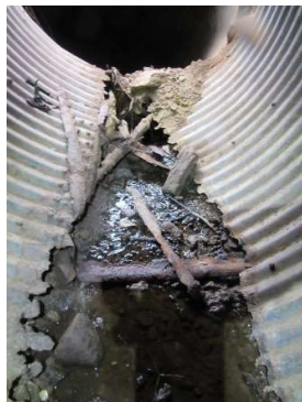
Severe corrosion to invert of Armco culvert
