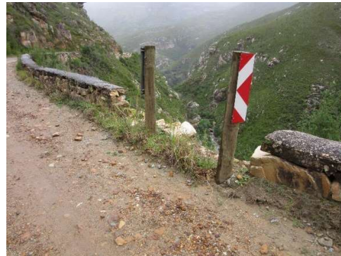
Damage to dry-stack balustrade wall on DR1640 at km 7.55
