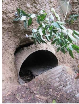
Downstream section of the Armco culvert washed away and collapsed due to erosion
