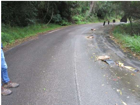
Road slip on RHS at MR00355 at km 7.95
