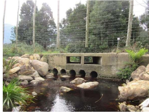
Downstream – looking towards culvert. Flood fence missing.
