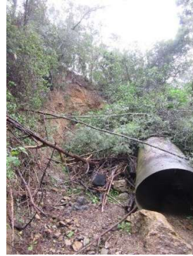
Downstream section of the Armco culvert washed away and collapsed due to erosion
