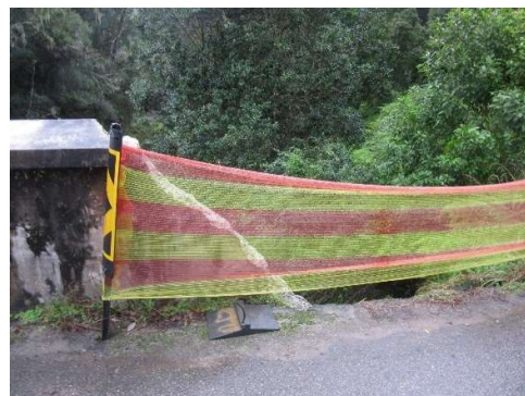
One of the end-blocks and part of the balustrade to the Salt River bridge on road MR00355 at km 8.67 was knocked down by vehicle impact. This is on the RHS when approaching the bridge from Saasveld side.
