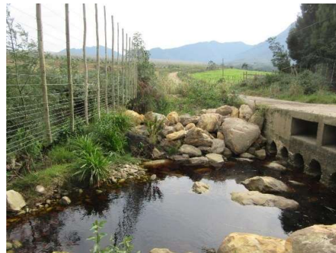
Rip rap has recently been placed on the downstream side to reduce scour
