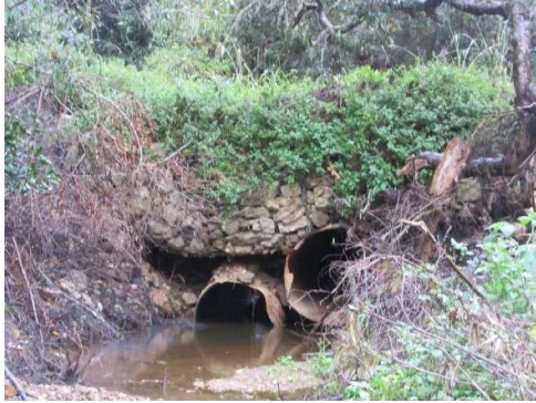
Existing Armco culvert on private road upstream of MR00355 at risk of collapse. May cause damage to MR00355 if this happens.
