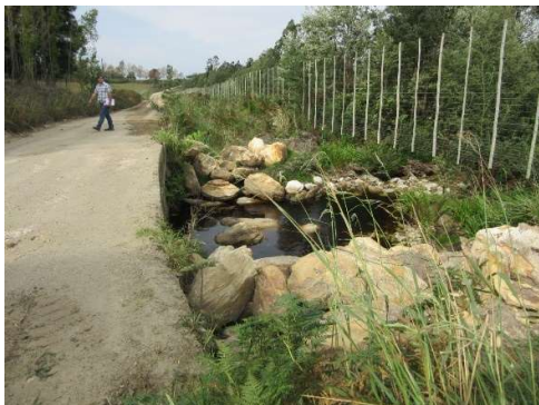
Rip rap has recently been placed on the downstream side to reduce scour
