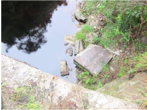
Remains of the damaged end-block and balustrade
