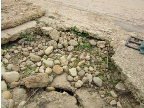
Damage to deck and pipe culvert caused during previous flood.
