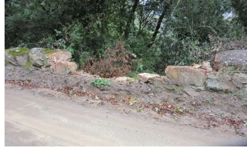
Damage to dry-stack balustrade wall on DR1640 at km 9.84
