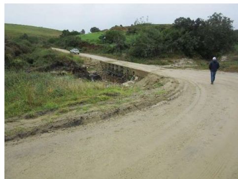
During the November 2021 flood the George side approach road was washed away for a length of 15m. This portion of road has been repaired and widened
