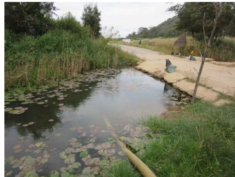
Water ponding downstream of drift
