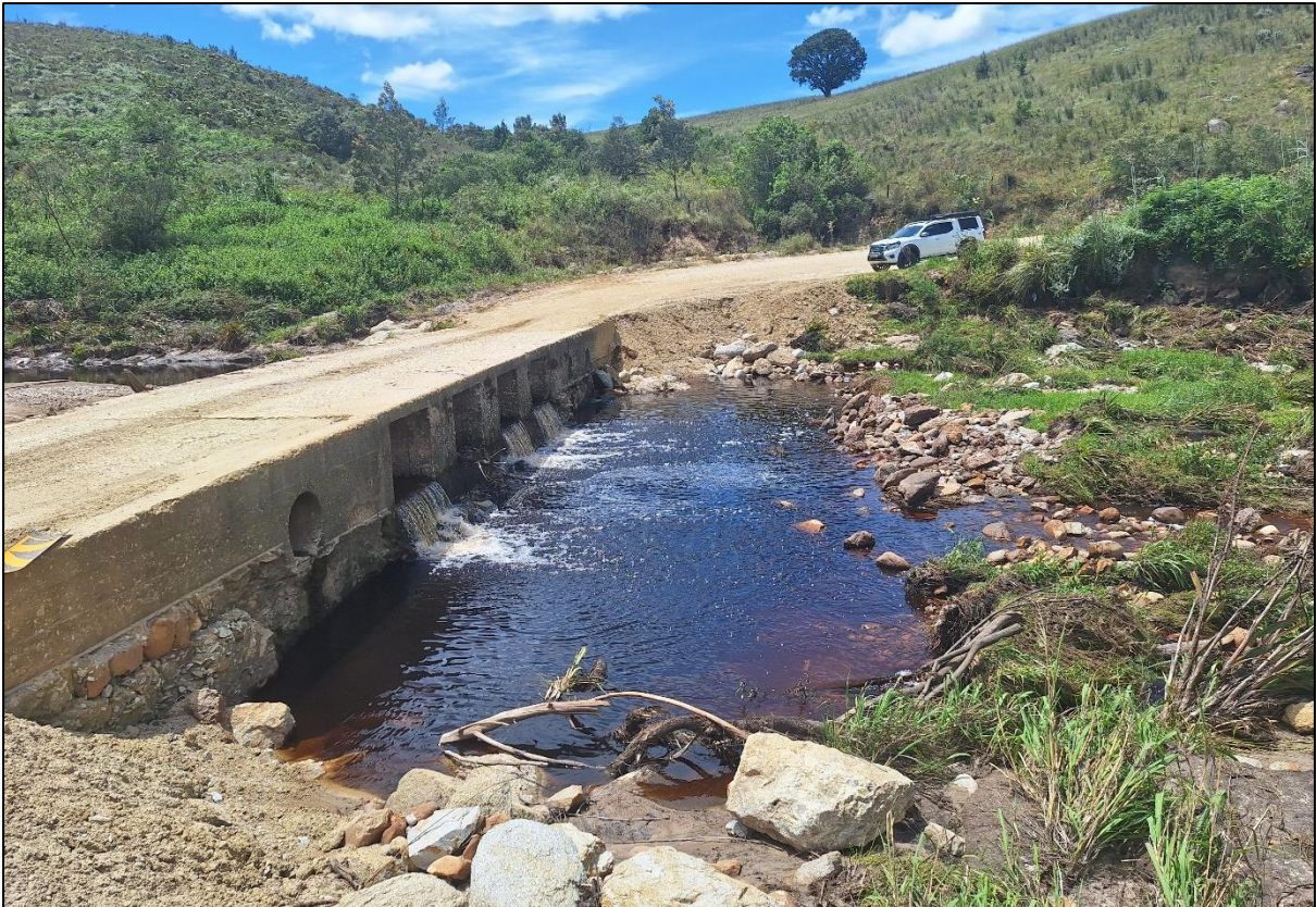
Plate 10: Photograph showing the culvert confining flows resulting in scouring of the river bed downstream and erosion of the banks
