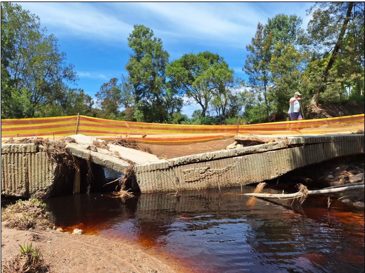
Plate 1: Photograph of the collapsed Site 4 causeway on the DR1633 Jonkersberg Road (km 3.35) over the Varings River in Jonkershoek
