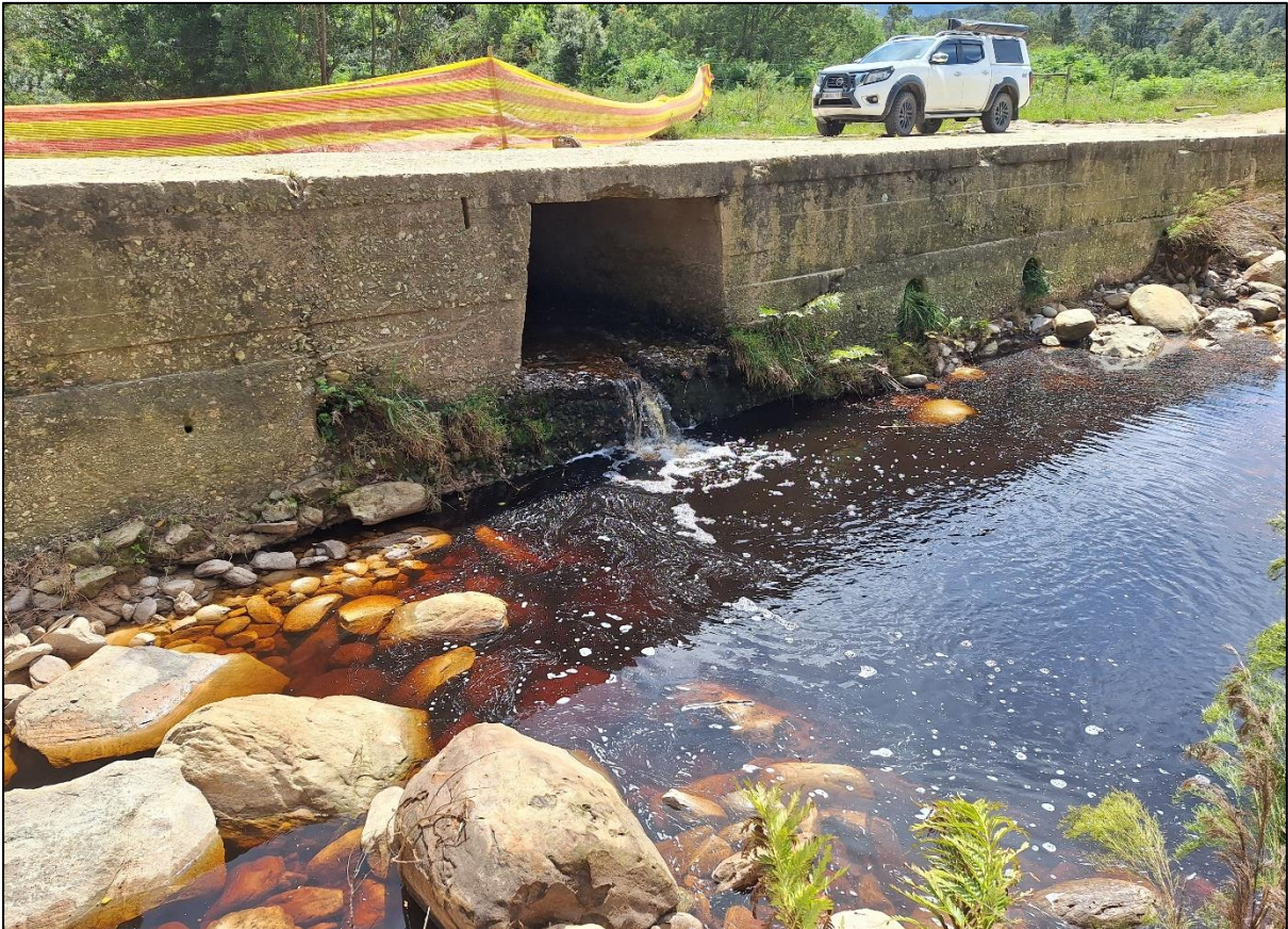
Plate 7: Photograph of the single small culvert at the site 4 causeway resulting in confined flow and scour downstream
