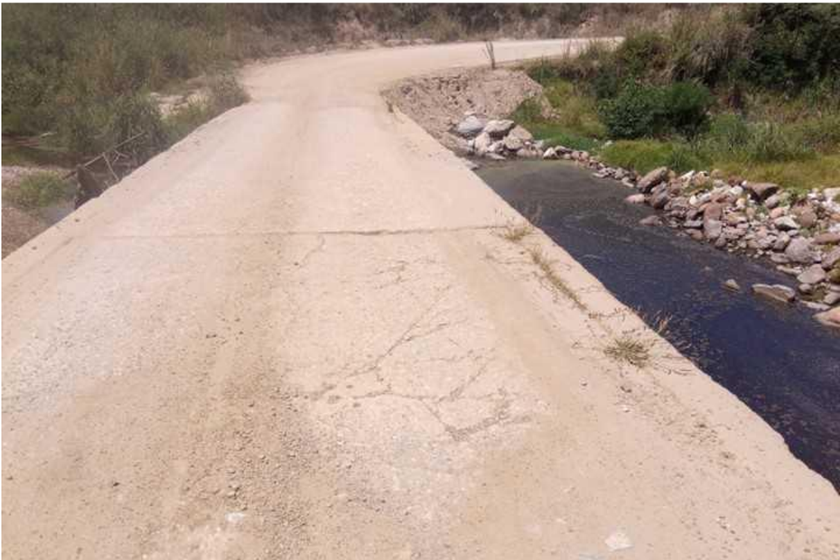
Figure 7. Site 8 - showing the causeway and damage.
