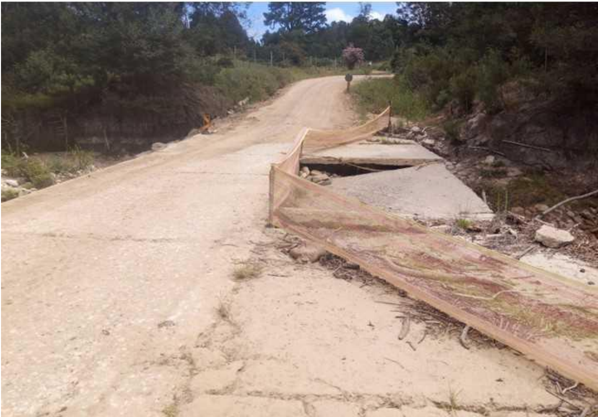
Figure 5. Site 4 - showing the causeway, flood damage, and immediate surroundings viewed from the West (top) and viewed from the East (bottom).
