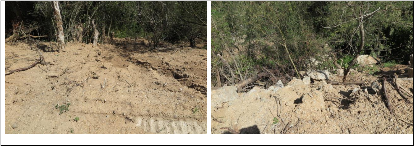
The last two images above show erosion gullies starting to form on the un-stabilised cut slopes.
