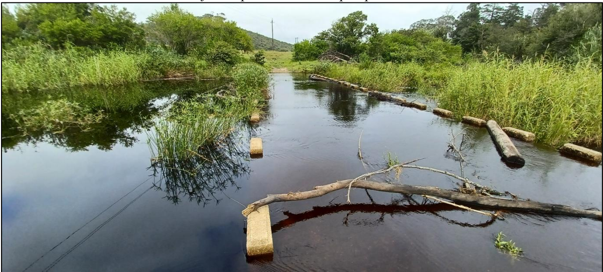
Plate 3: A photograph taken of the old road crossing the Moordkuil River, which acts as a weir for the pumpstation
