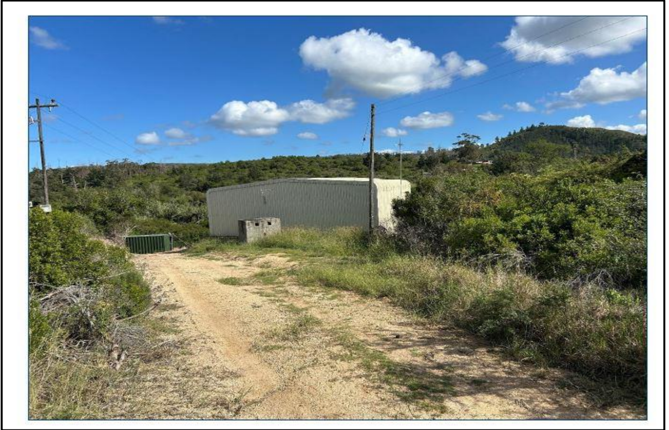
Figure 8: Thicket on eastern side of pump station and position of temporary access to construction site.
