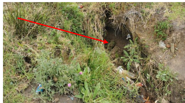
Figure 42: Eroded and polluted watercourse.
