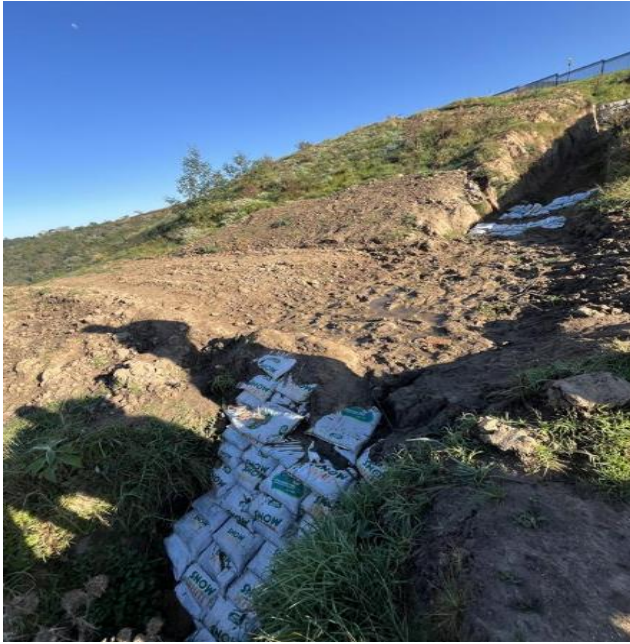
Figure 5: Angle from downstream of diverted stormwater outlet route with erosion gully formed. Access road traversing flow path. The estimated depth of existing erosion gully is approximately 2 – 2.5m deep.
