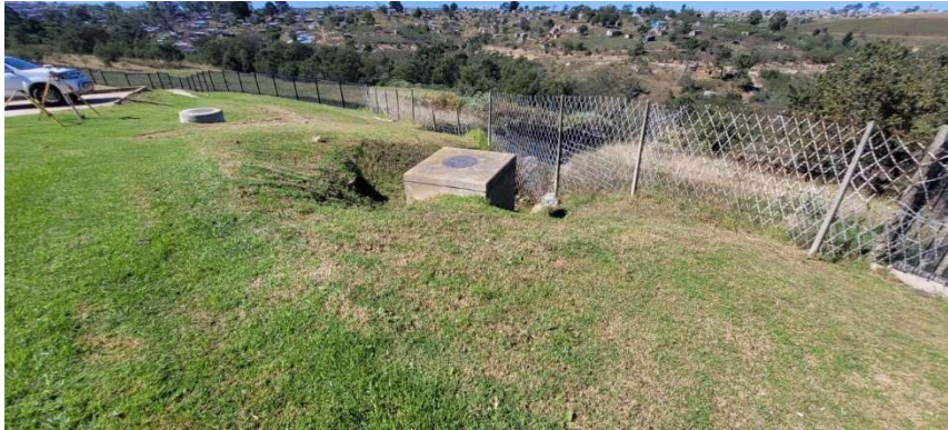
Stormwater outlet that started eroding (photograph taken April 2020)
