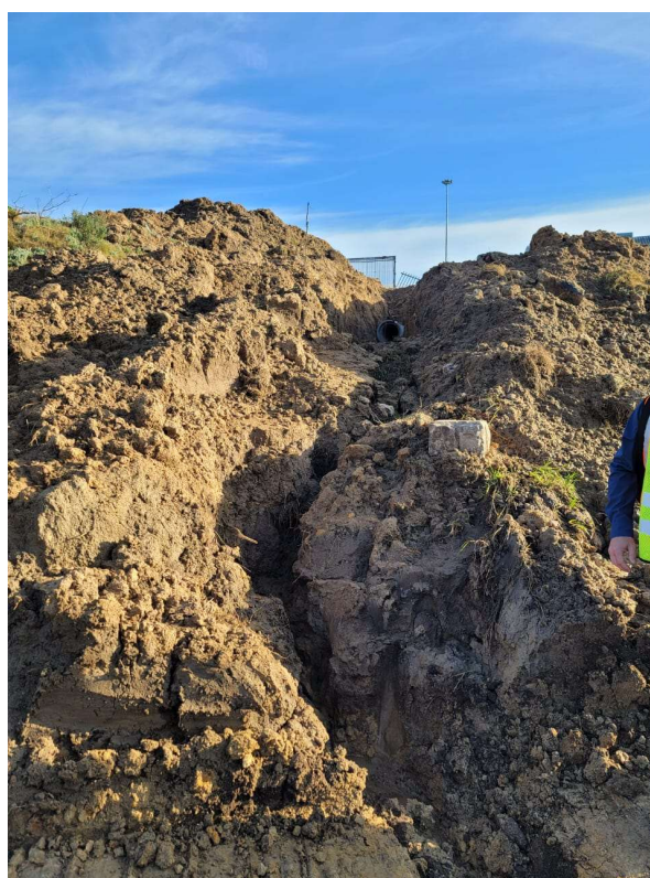
Point at which the diverted stormwater is currently released and that is eroding (photograph taken July 2023)
