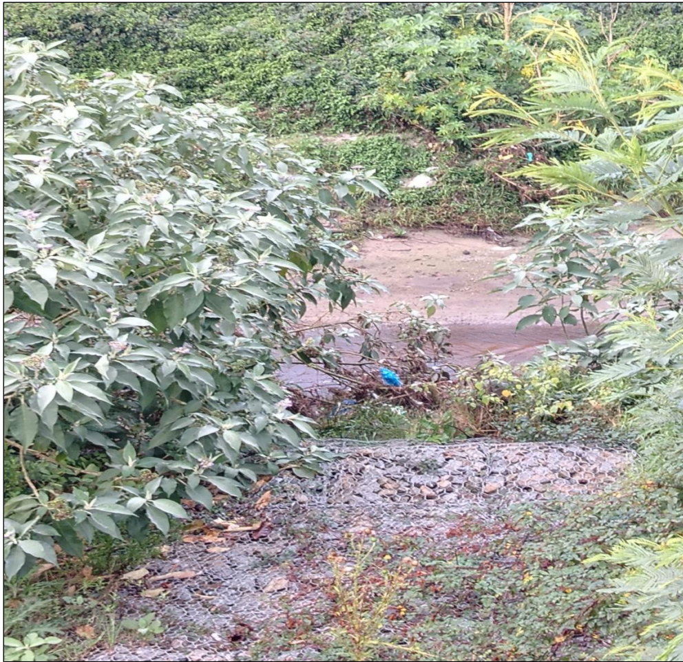
Image 13: Close-up view of the gabion discharge point (Dense stands of mature Solanum mauritianum (Bugweed)).
