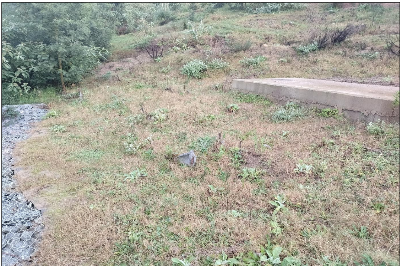
Image 12: Photographic evidence of alien plant recruitment on the rehabilitated embankment.
